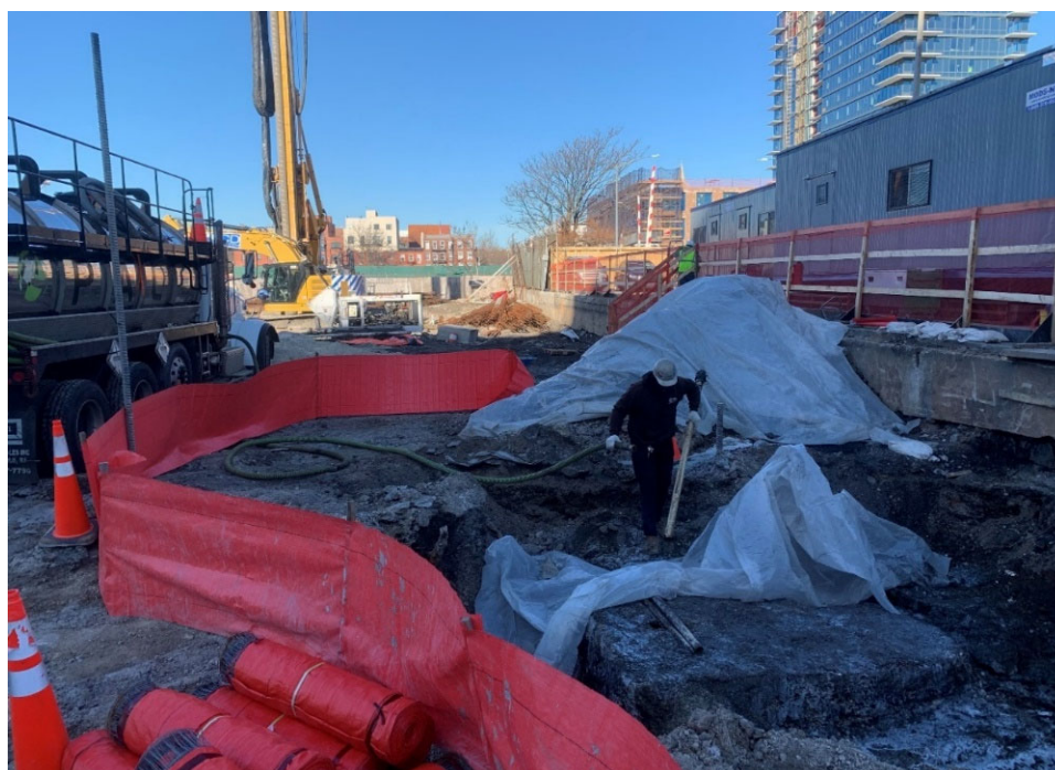
Photograph No. 8: Representative photo of PAL pumping out Tank-11 on 2/7/24.
