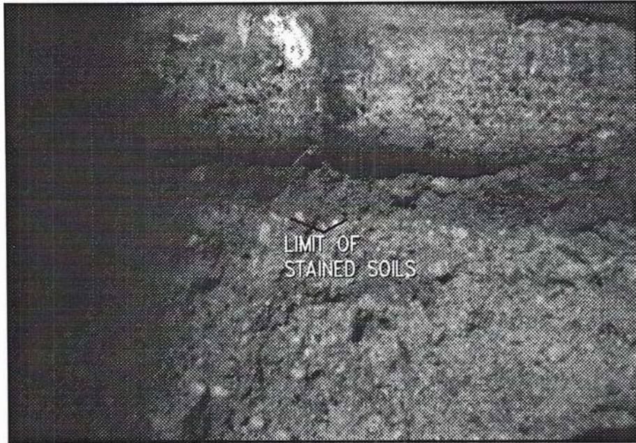
Figure 3. Cracked joint on 4" \varnothing transite drain line and limits of stained soils.
