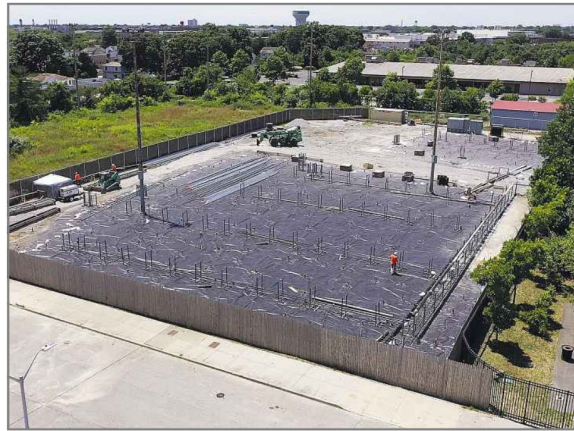
Work is being done June 26 at the Bethpage Ballpark, which was once a dumping ground for a nearby Grumman facility.
