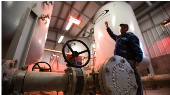
Brookhaven Science Associates environmental engineer Vinnie Racaniello at the North St. groundwater treatment system in Manorville on Mar 13, 2020. Credit: Jeffrey Basinger
