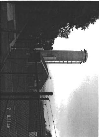
4. Existing Air Stripper Tower at Bethpage Water District-Plant #4
