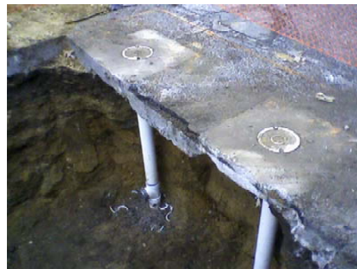
Connections to depressurization wells
