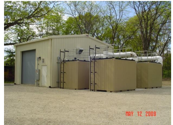
Completed treatment building and ECUs
