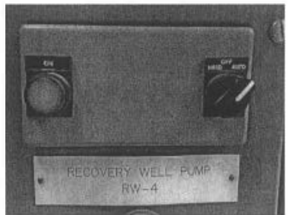
Recovery Well "HAND-OFF-AUTO" Control
