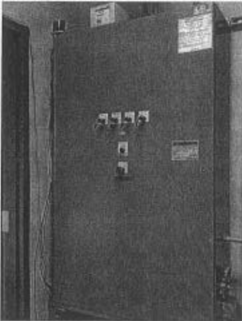
Recovery Well Pressure Switch Control Panel
