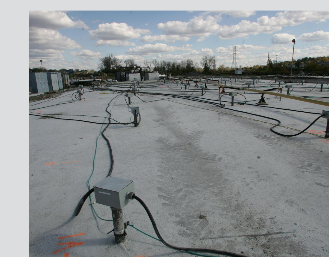
ISTD Wellfield during Operation
