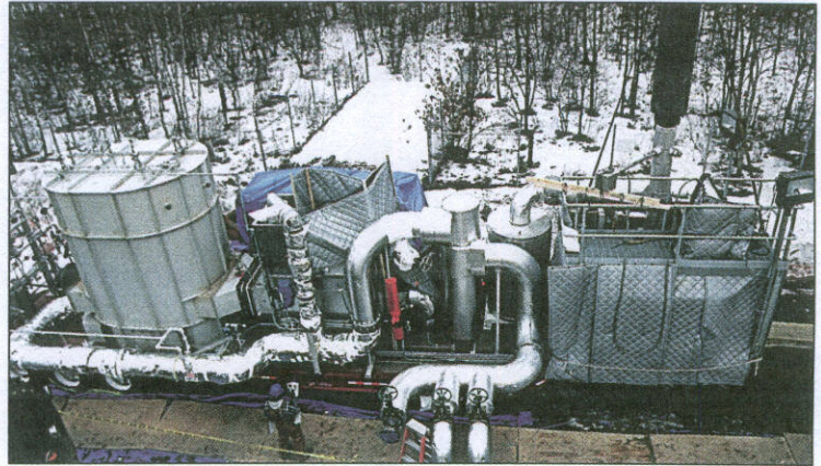
Mobile Vapor Treatment System
