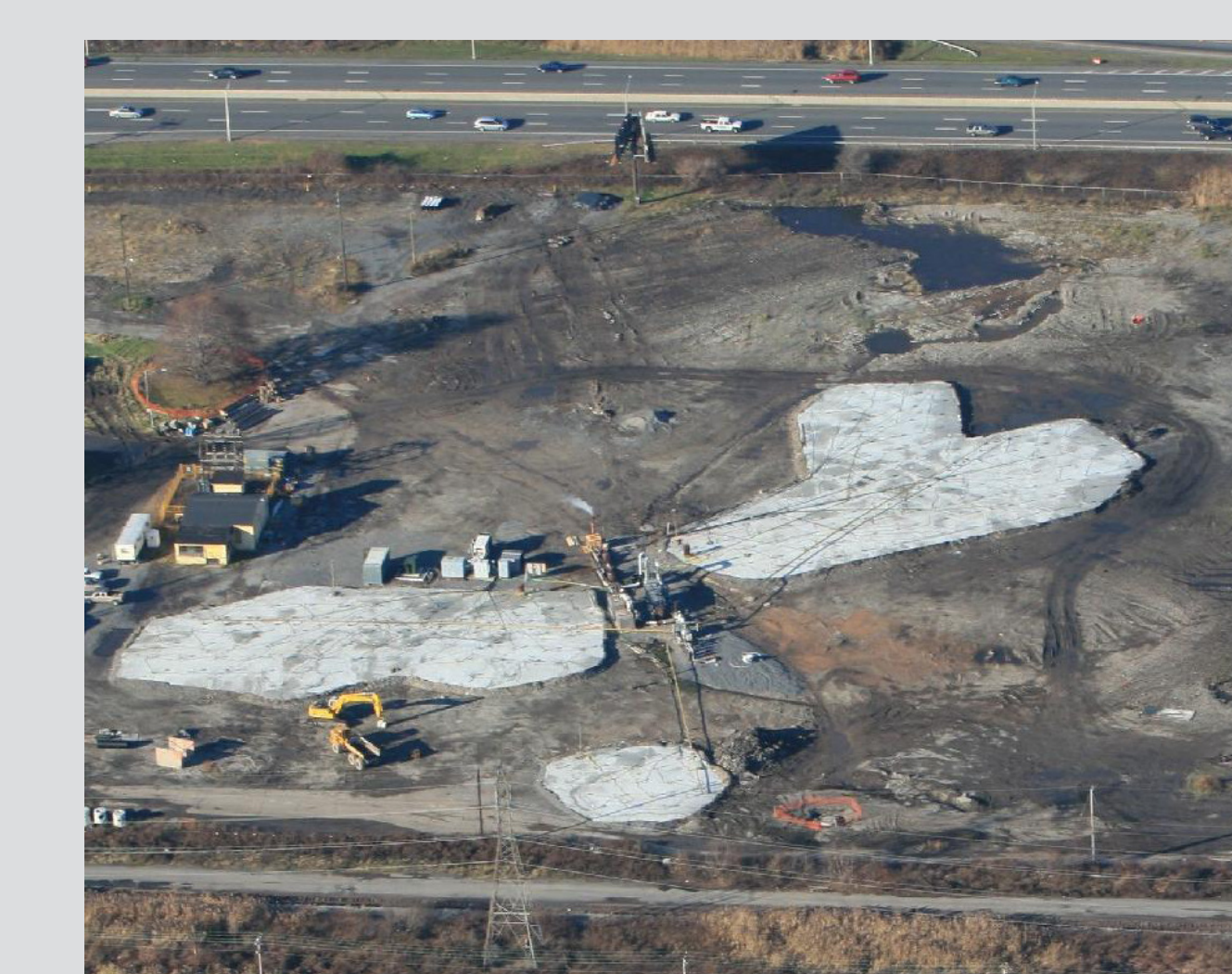
ISTD System during Operation
