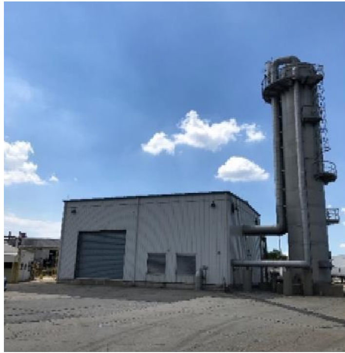
Typical Large-Scale Treatment Plant
