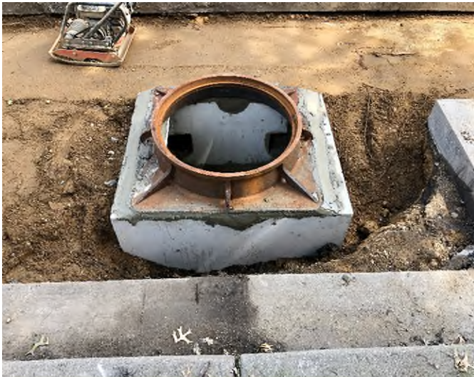
Electric vault along Grumman Road East
