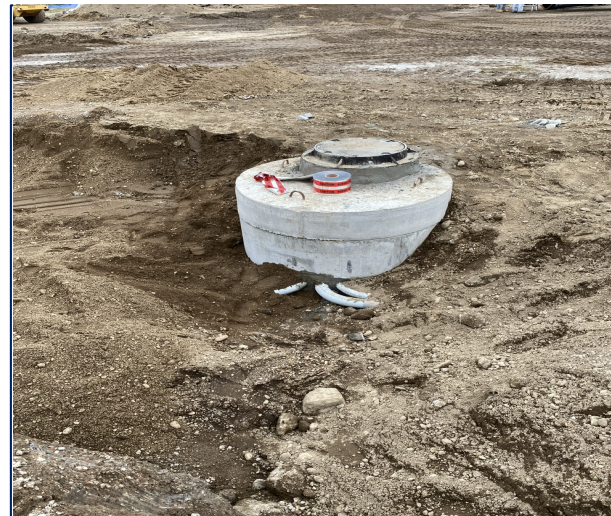
Leak Detection Manhole for Influent Pipeline
