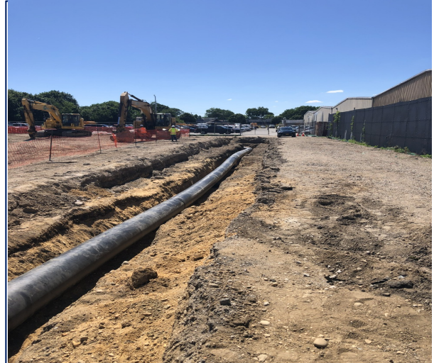
Installed Influent Pipeline
