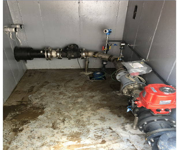
Piping Inside RW-22 Vault
