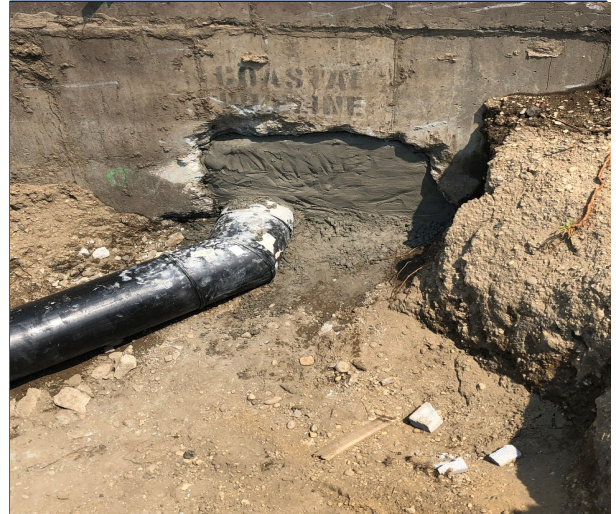
Effluent Pipe Connection to Control Structure B
