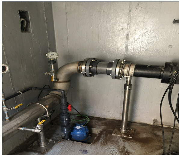
Piping in RW-20 Vault
