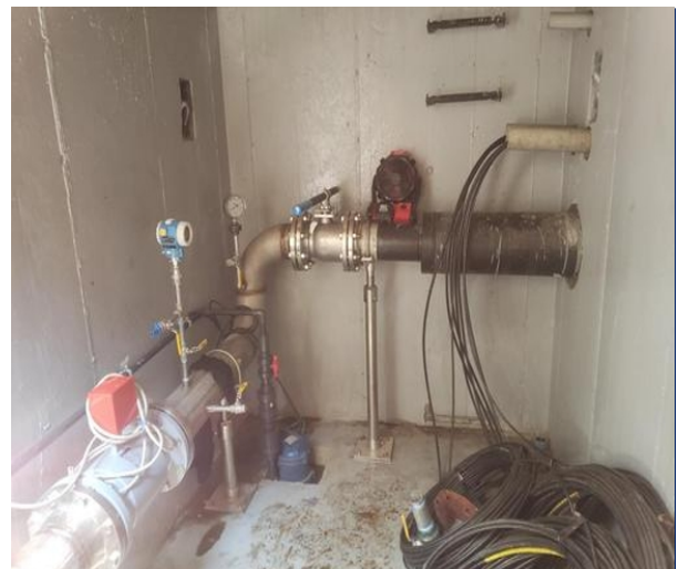
Piping in RW-20 Vault
