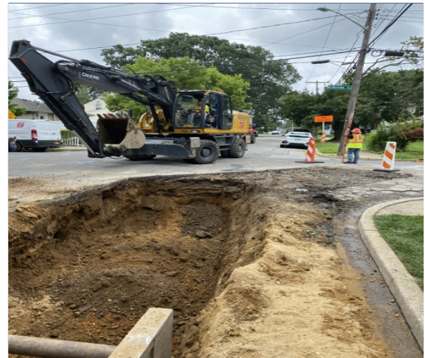
Excavating Pipe Trench at Corner of Sophia St and N Herman Ave
