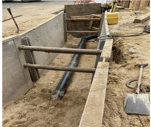
Installing HDPE Pipe at Corner of Sophia St and N Herman Ave
