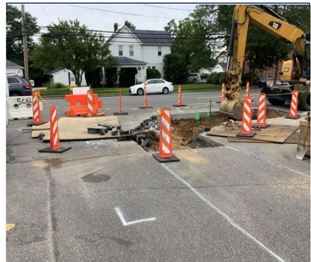
Excavating Pipe Trench at Corner of S Pershing Ave and Stewart Ave
