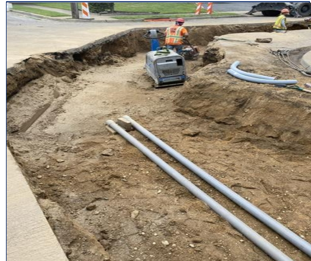
Installing PVC Leak Detection Conduits at Corner of Sophia St and N Herman Ave
