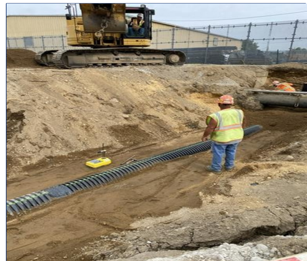
Compaction Testing of Piping Trench between Manhole MH-1 and Catch Basin CB-2
