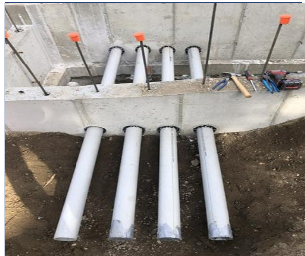
Conduits for Incoming Electrical Service on South Side
