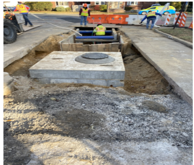
Air Release Vault Structure on S Sheridan Ave
