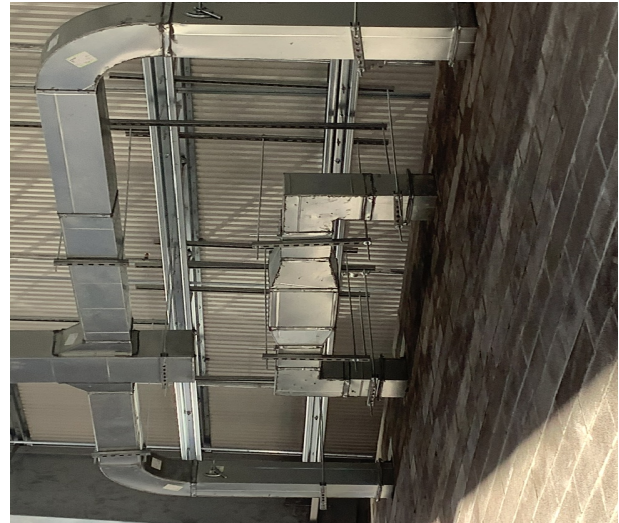
HVAC Ductwork and Sprinkler Piping
