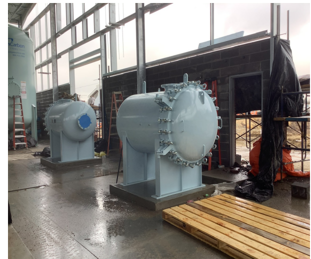
Cartridge Filters Placed on Concrete Pads
