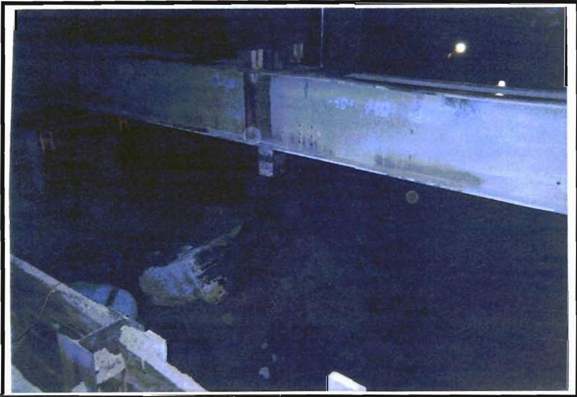
Photo 4: Demolition of Building Column Footer. Needle beam in place to support column.
