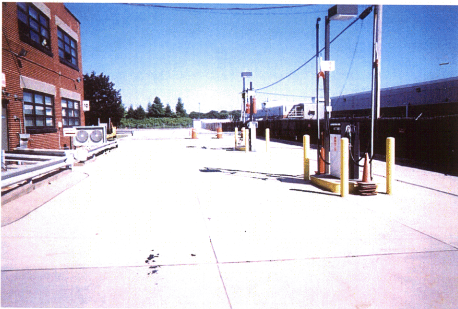
Photo 2: Fuel Pumps on South Side of Building 20-01
