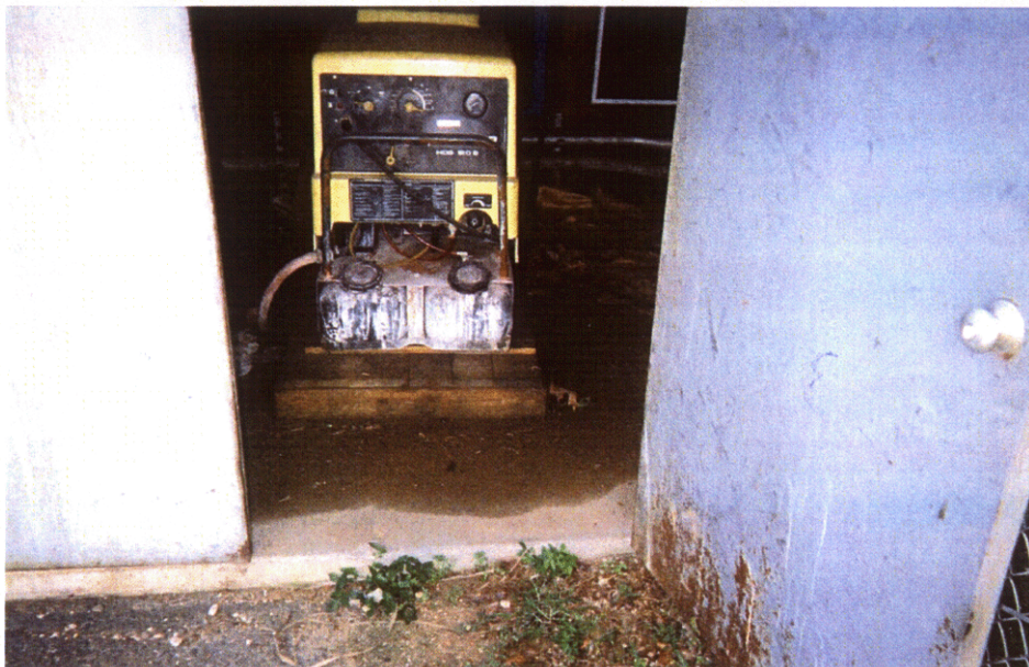
Photo 7: Steam Jenny in Building 20-03
