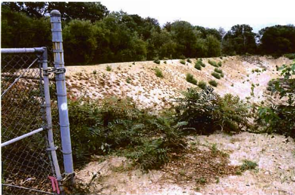
Looking N at berm north of recharge basin. Samples BP-S2-278 through 280 were taken here
