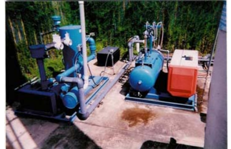
Air sparging uses air to help remove chemical vapors from both soil and groundwater. The soil vapor extraction system then works like a vacuum to extract and collect the volatile chemicals for proper disposal. AS/SVE systems work best on volatile chemicals, like those found at NWIRP, Site 1 (“Former Drum Marshalling Area”)
