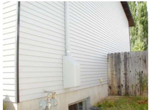
A sub-slab depressurization system is an effective, proven way to keep chemical vapors from entering the indoor air of homes. A pipe is installed below the basement floor and connected to a blower. The blower pulls the vapors from the ground before they can enter the home and vents them outside.
