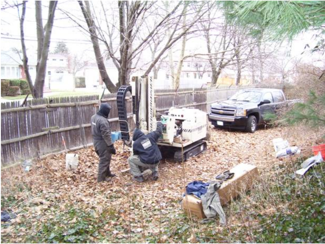
Site 1 - Eastern Fence Line, looking southeast – Location of SVE Wells
