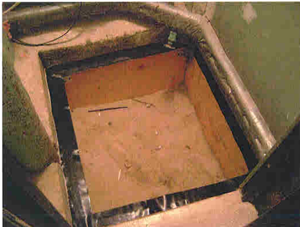
Photo 17: Home #4 sump before being sealed.
