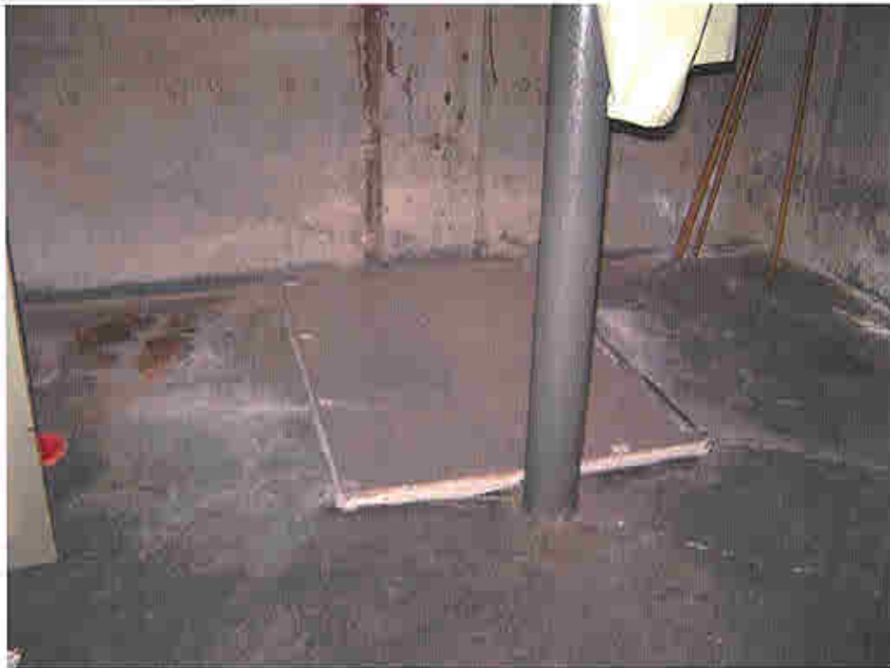
Photo 12: Sealed sump at Home #3.
