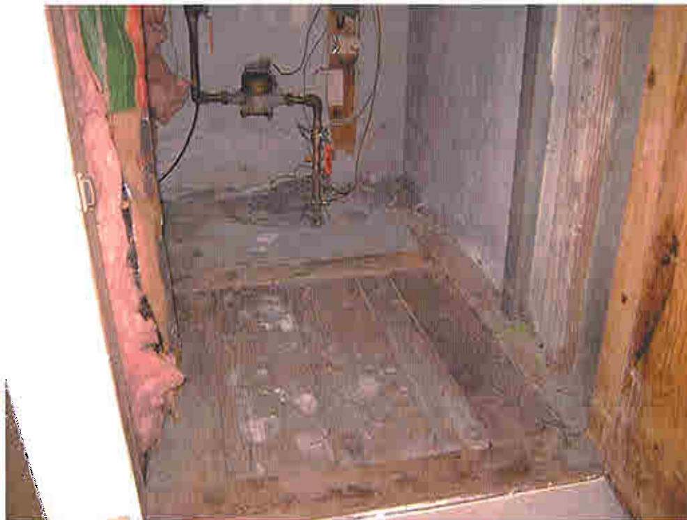
Photo 6: Home #2 sump before being sealed.
