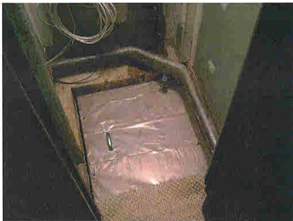
Photo 18: Sealed sump at Home #4.
