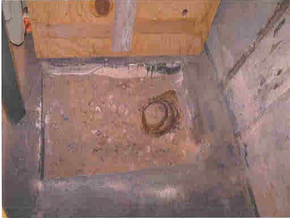
Photo 11: Home #3 sump before being sealed.
