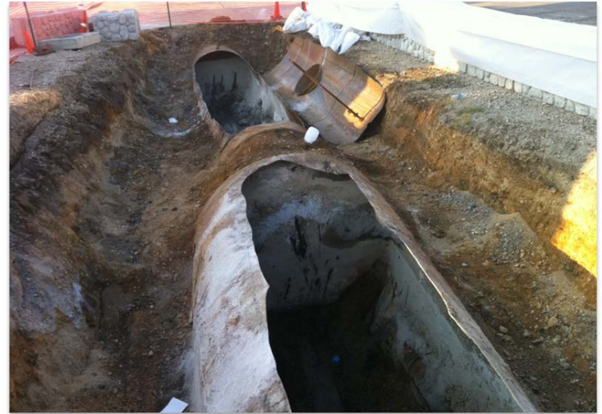
Condition Post Removal of Fluid and Sediment
