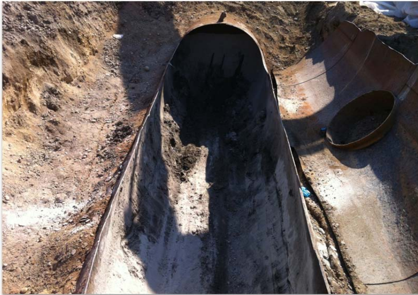
Condition Post Removal of Fluid and Sediment
