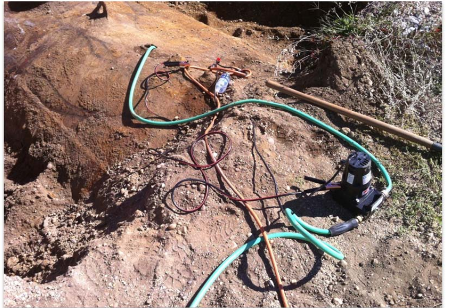
Pump set-up for Fluid Removal
