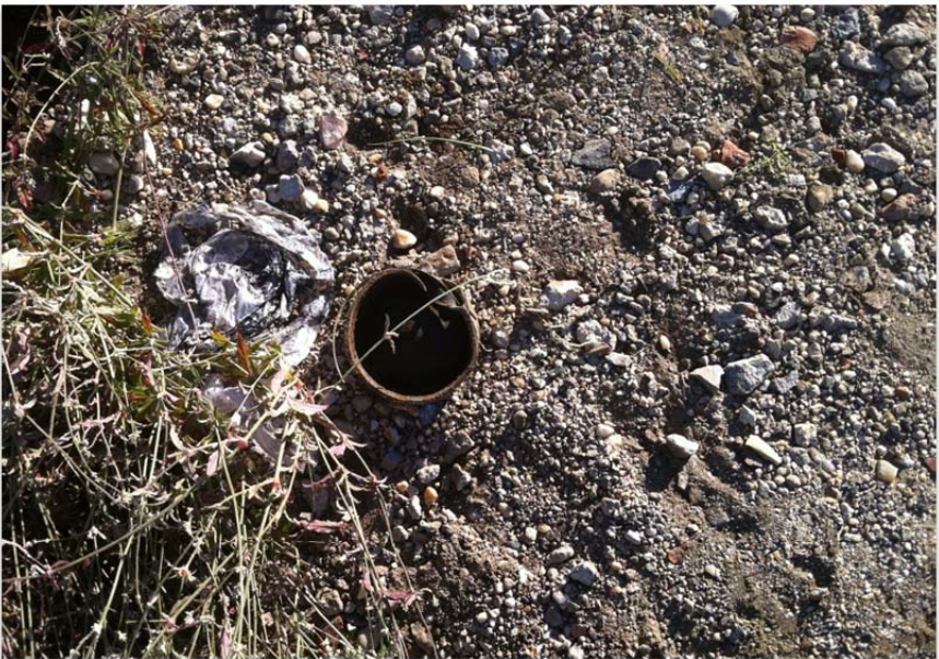
Tank Vent Pipe
