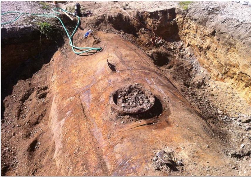
Removal of Fluids
