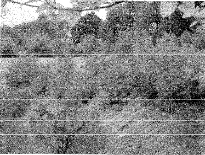
Erosion east side of Southern Basin – Site 2
