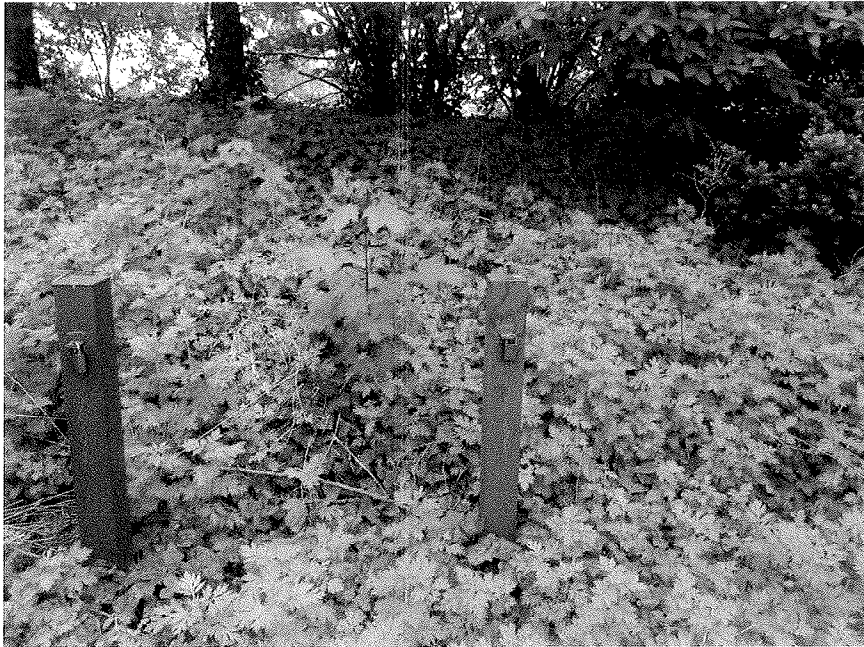
Soil vapor extraction wells 103I & 103D – Site 1
