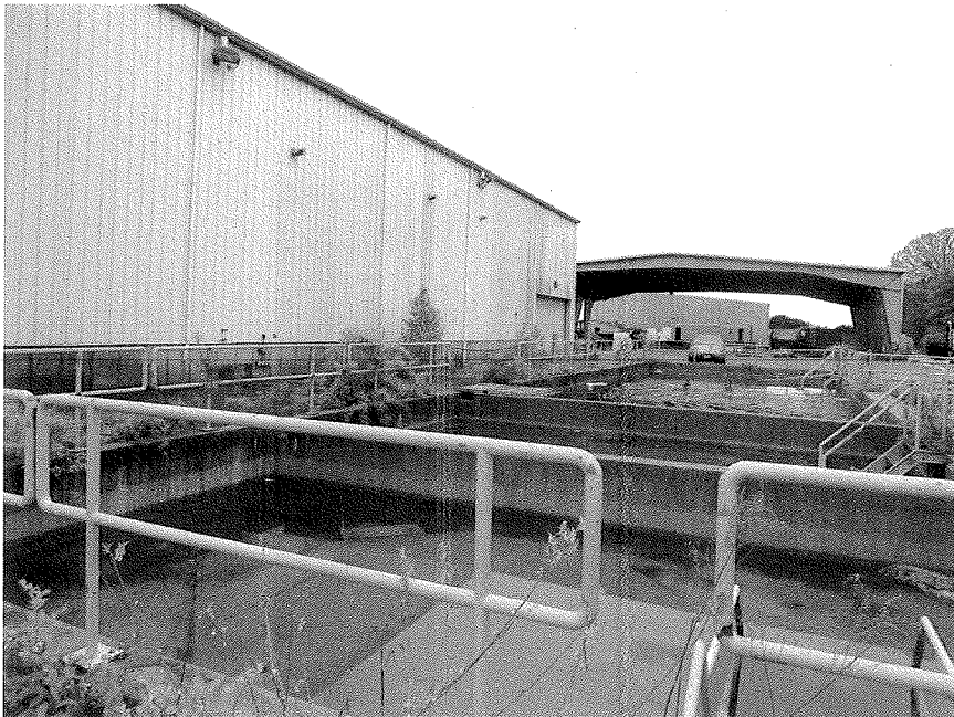
Secondary containment for county waste water treatment tanks – Site 2
