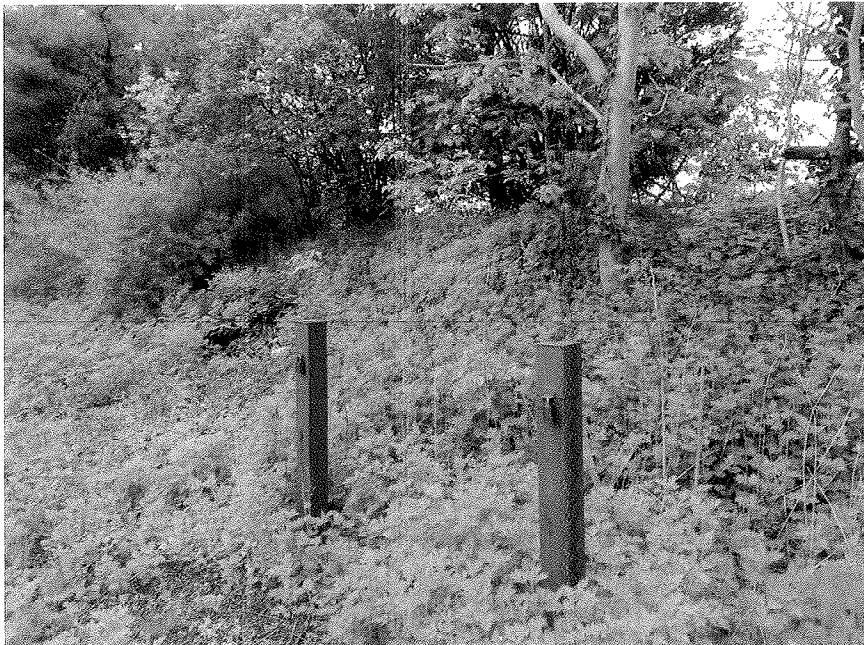
SVE extraction wells 104 I&D – Site 1
