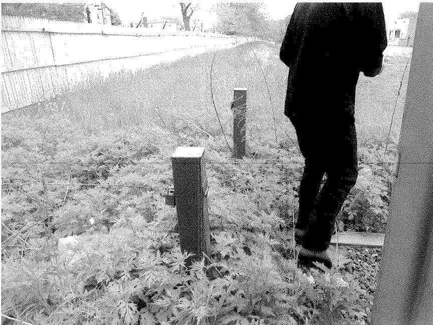
Soil vapor extraction well 102D – Site 1
