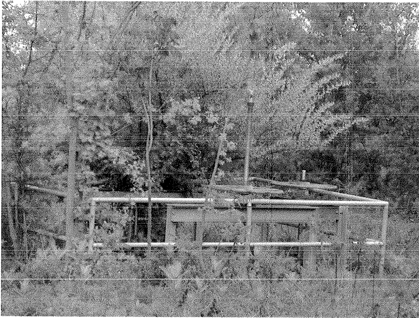
Valve Distribution Box for OU3 recovery system – Southern Basin Site 2
