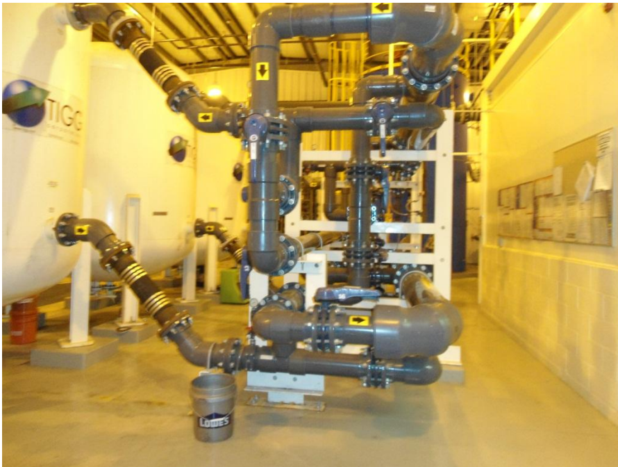
GM 38 Pumping system – OU2
