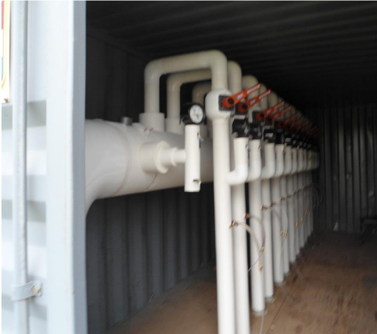
SVE header system – Site 1
