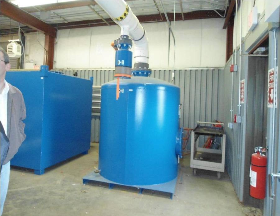
Condensation Tank – Site 1 SVE system
