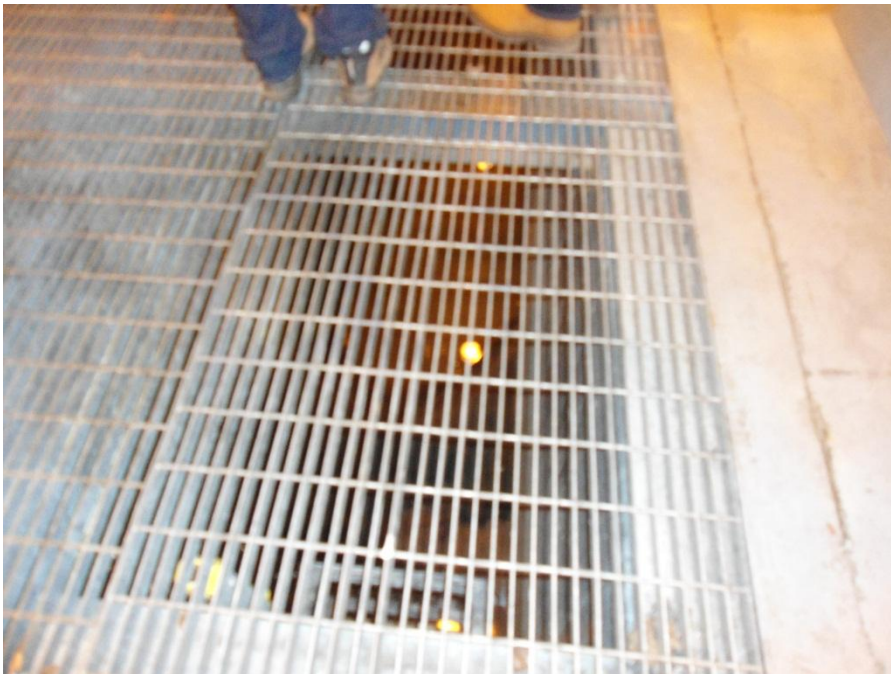
Grate area, GM38 operations room – OU2
