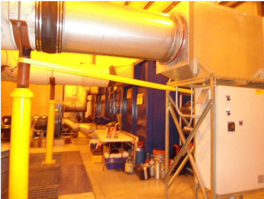
GM 38 Main operations room – OU2
