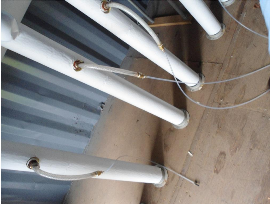
SVE lines and manifold – Site 1
