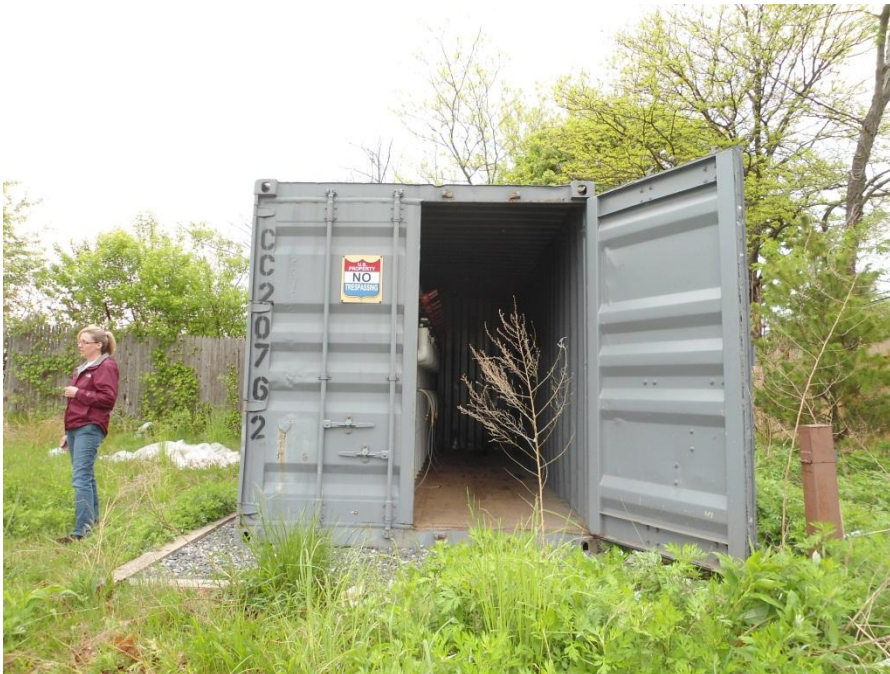
Conex Box that holds Site 1 SVE manifold – Site 1
