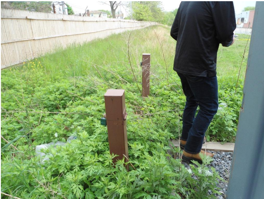
Soil vapor extraction well 102D – Site 1
