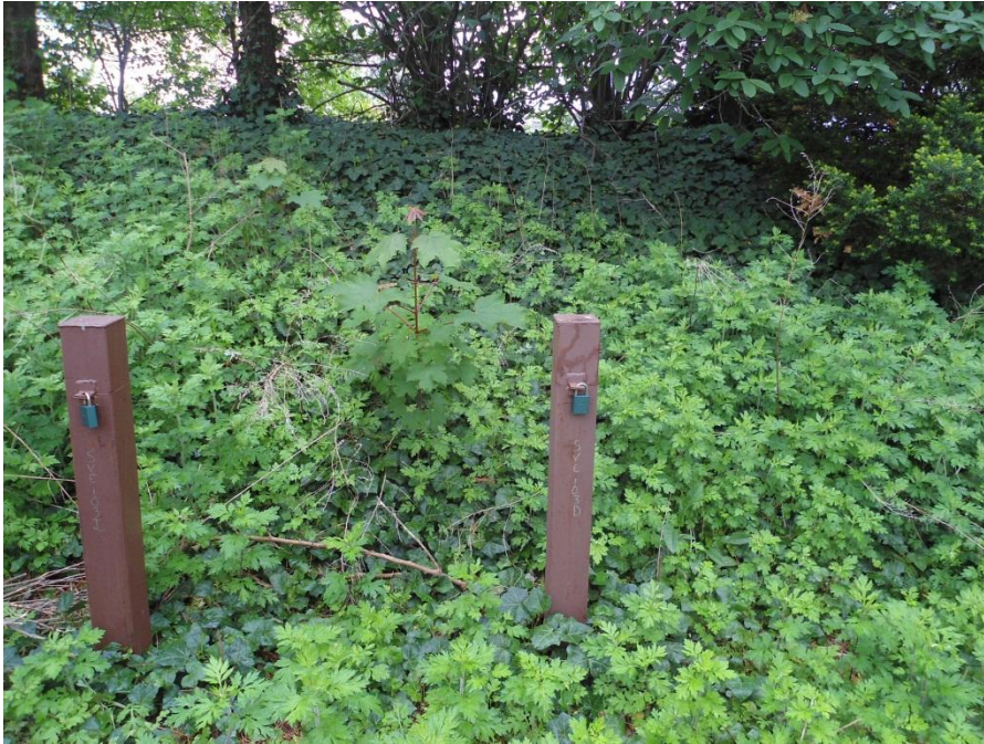
Soil vapor extraction wells 103I & 103D – Site 1
