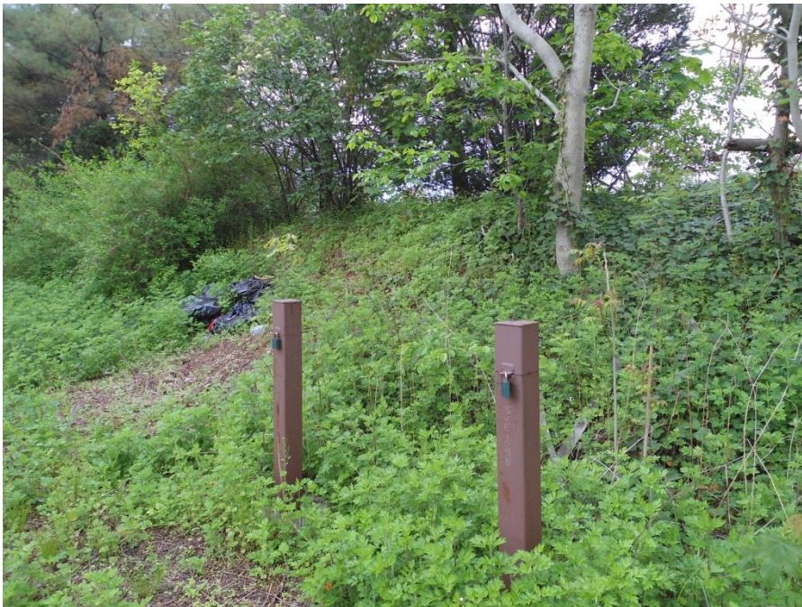
SVE extraction wells 104 I&D – Site 1
