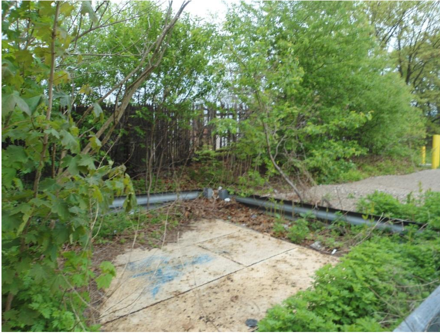
Water inlet for SVE system – Site 1
