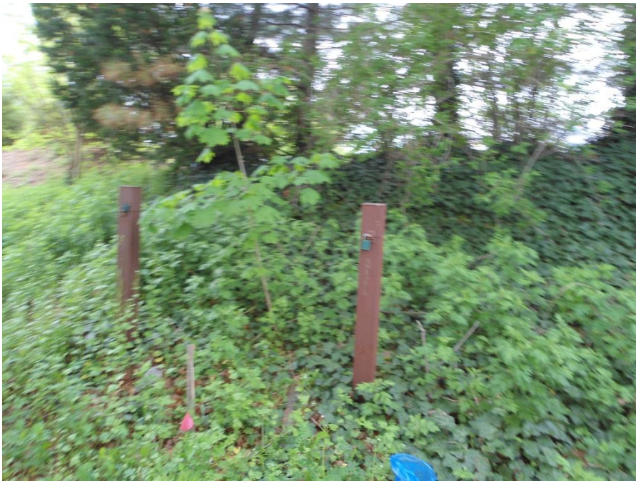
SVE extraction wells 102 I&D – Site 1
