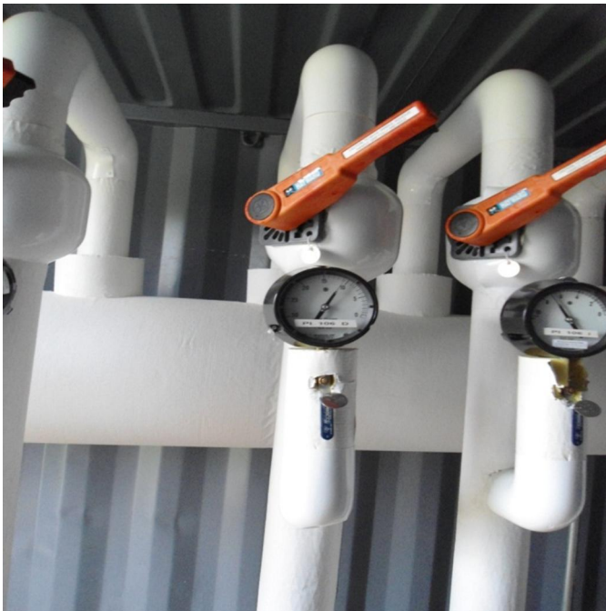
SVE lines and manifold – Site 1
