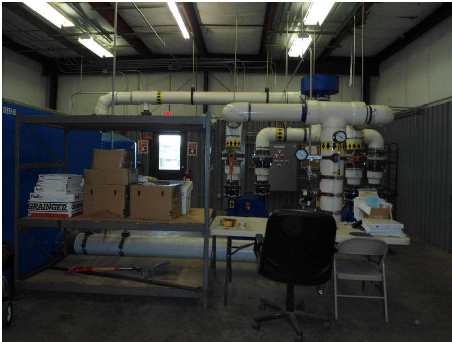
Site 1 Soil Vapor Extraction System
