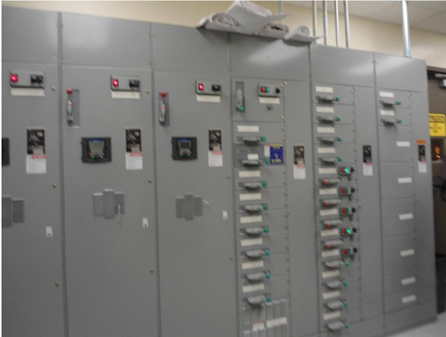
Control room GM-38 treatment system – OU2
