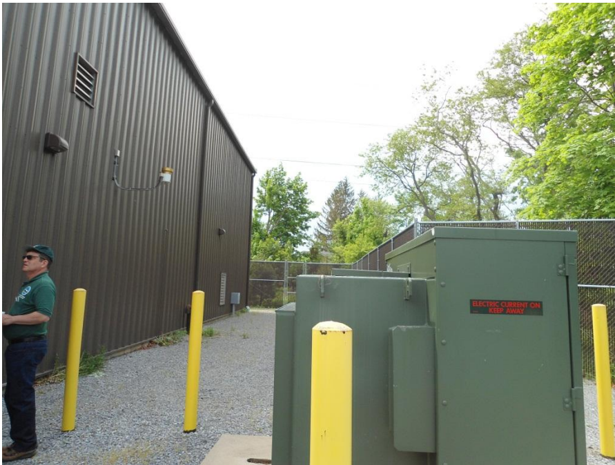
Outside GM 38 treatment system – looking south - OU2
