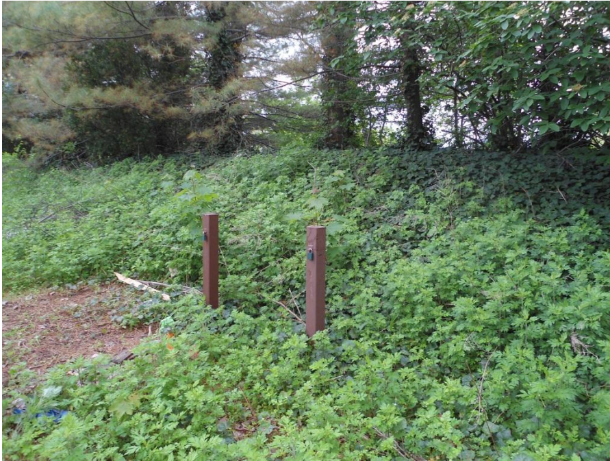
SVE extraction wells 103 I&D – Site 1
