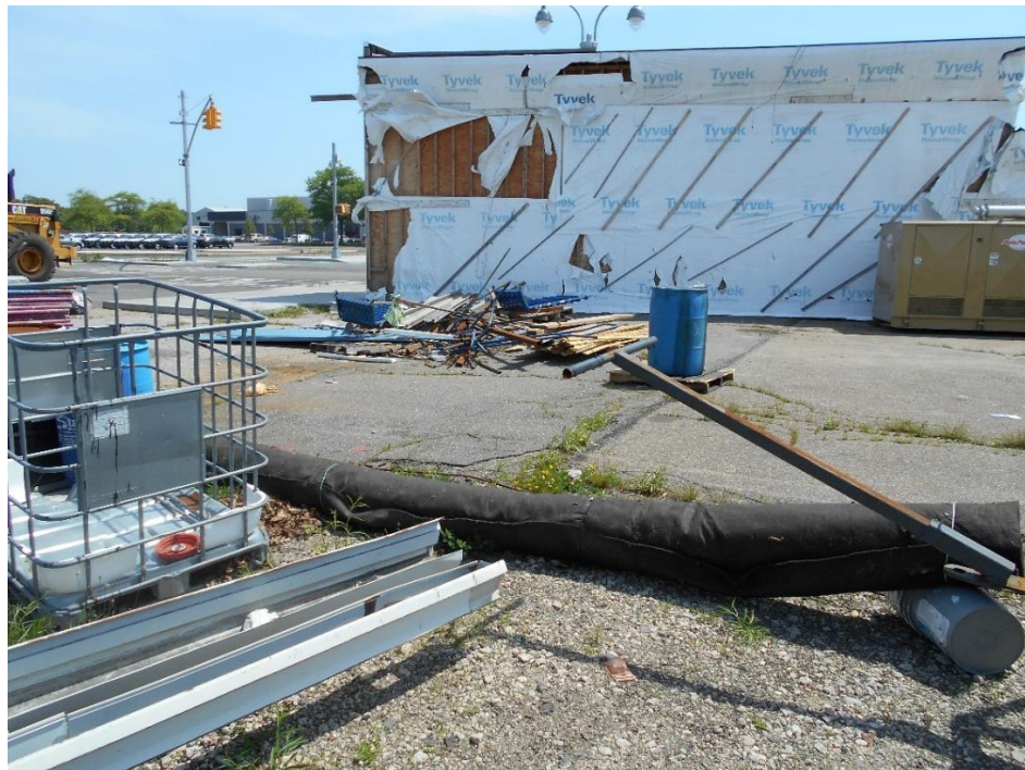
Photo 48: Site 3- Debris behind ticket booth
