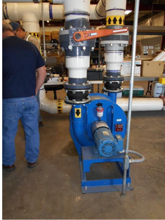
Photo 1: Site 1- Blower B-1A bolts missing
