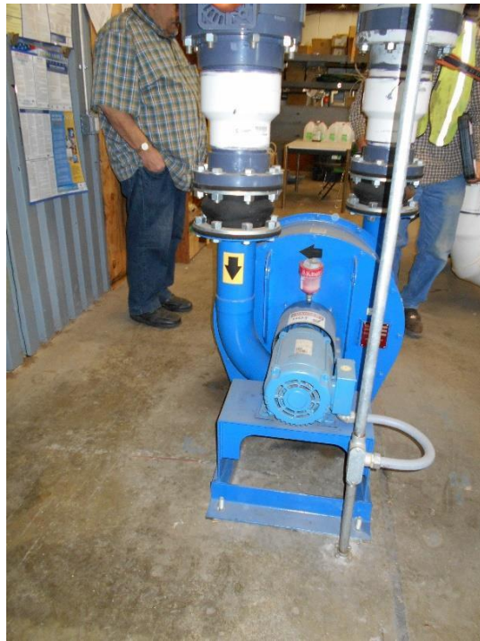
Photo 2: Site 1- Blower B-1B bolts missing
