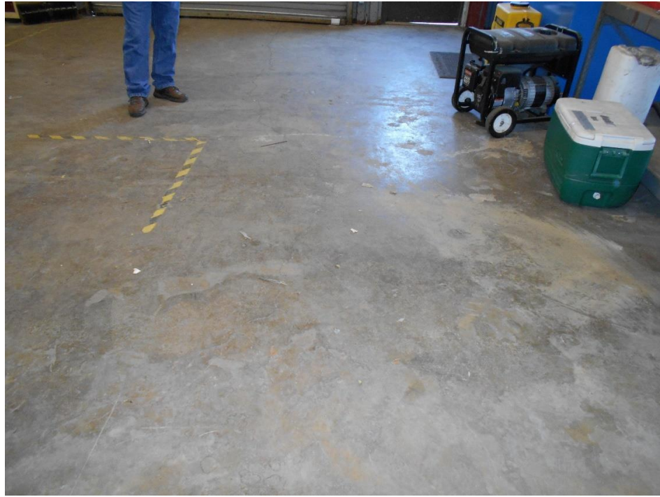
Photo 3: Site 1- Floor crack
