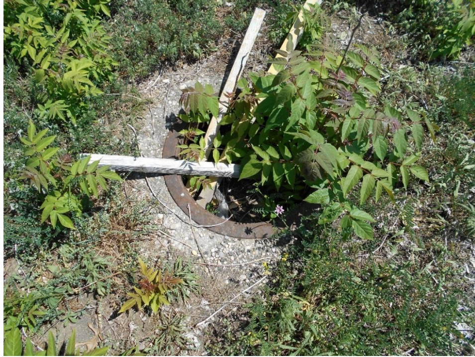
Photo 21: Site 1- Cesspool without lid
