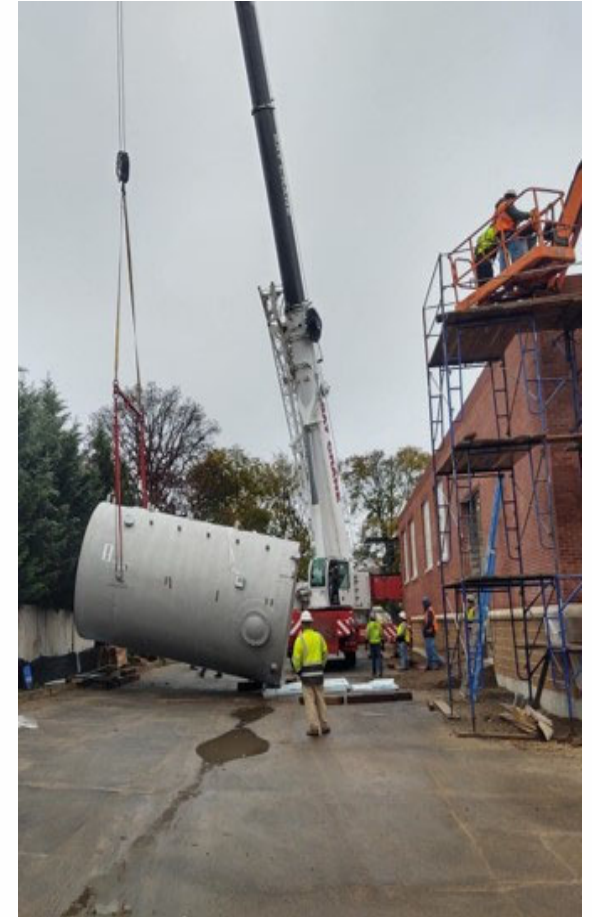
T-700, Backwash Tank
