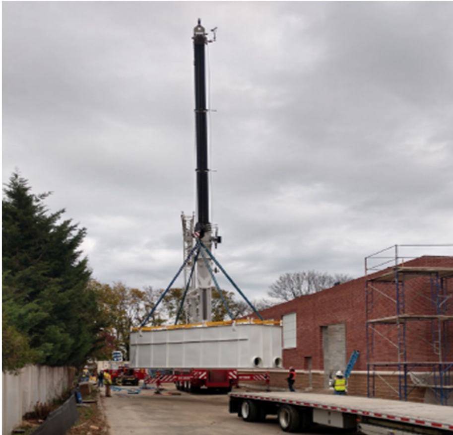
Vapor Granular Activated Carbon Unit
