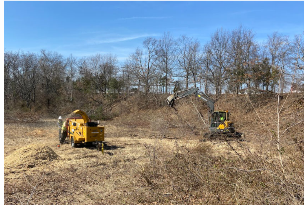
October 2022. Initial stages of clearing and grubbing within Nassau County Basin N477. Excavator being used to move cut organic debris to woodchipper. Looking north northwest.
