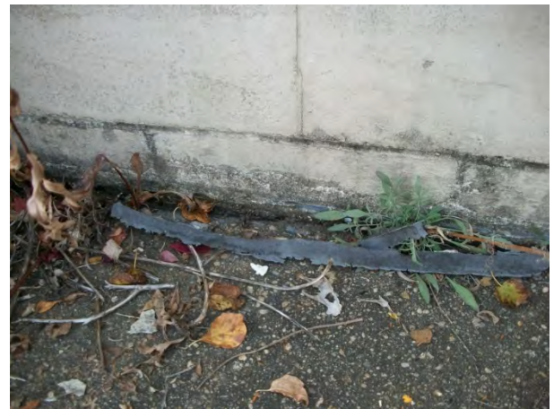
HA-23: Black Expansion Joint Caulking
