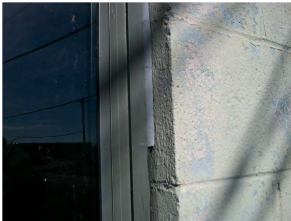
HA-22: Gray Exterior Window Caulking
