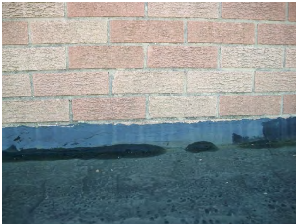
HA-33: Flashing Cement associated with North Entry Roof
