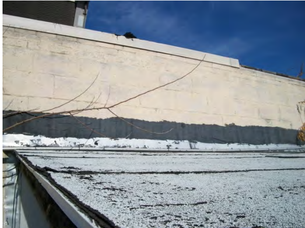
HA-31: Suspect Flashing Cement associated with South East Storage Roof
