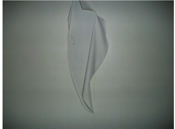
HA-19: White Joint Compound associated with HA-15
