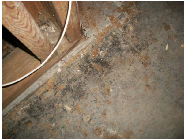
HA-14: Black Residual Floor Mastic
