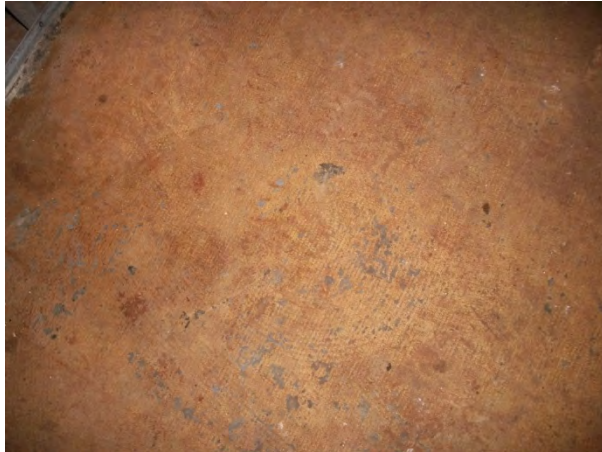
HA-18: Yellow Residual Floor Mastic
