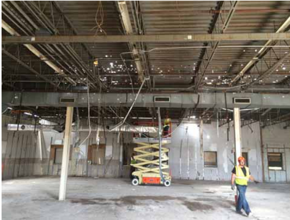
Construction and demolition debris removal activities in progress on the west side of the Administration Building interior.
