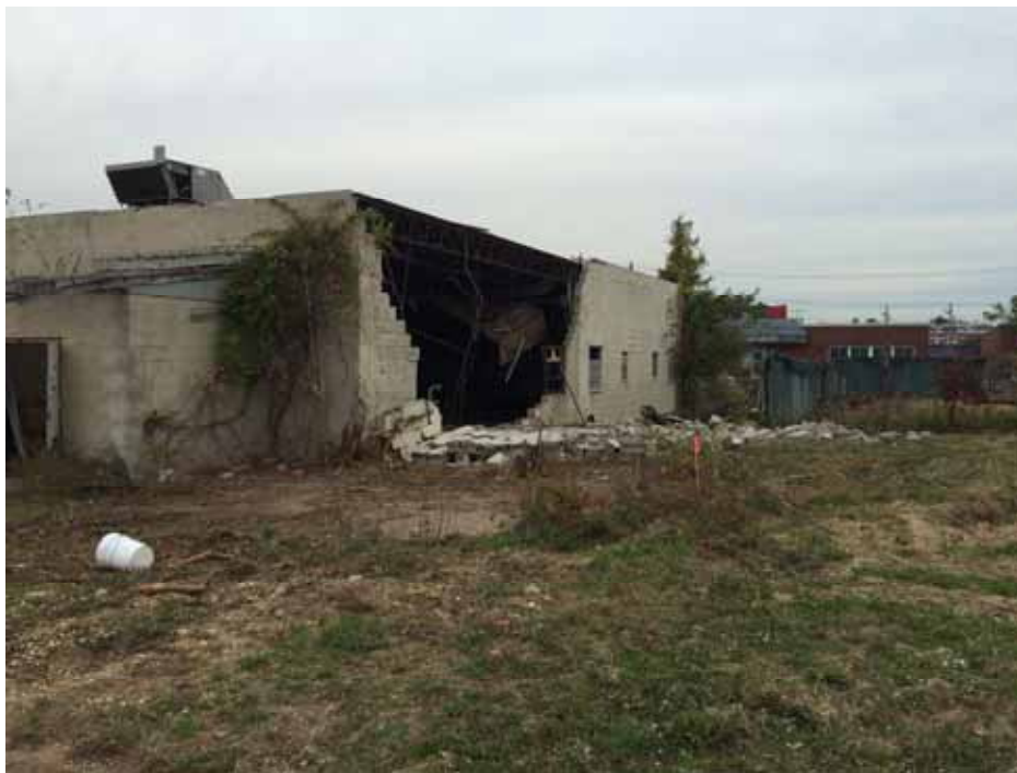
The east side of the Administration Building after the cinderblock wall collapsed outward.
