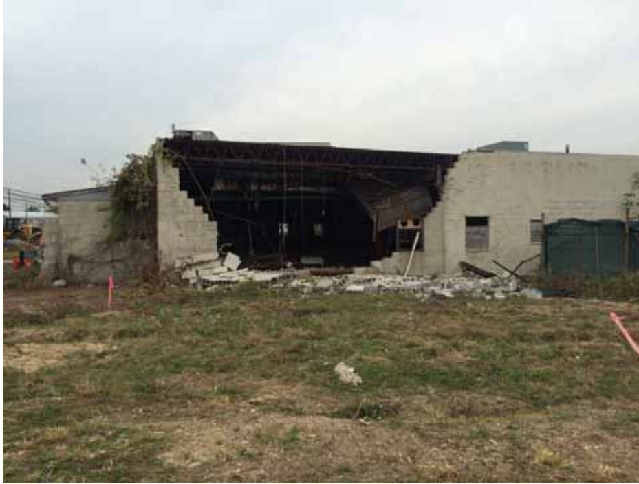
The east side of Administration Building after the cinderblock wall collapsed outward.
