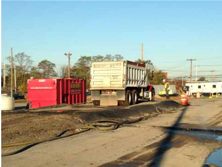
Posillico washing truck tires prior to leaving the site with non-hazardous waste soil.
