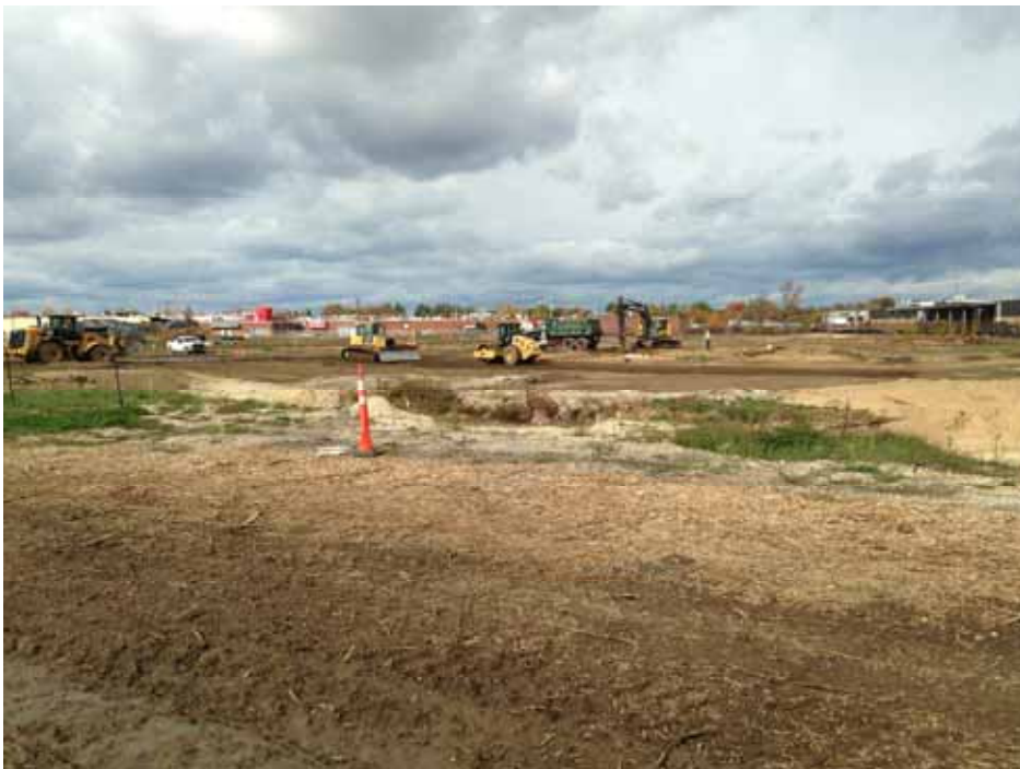
Posillico performing imported backfill material grading and compaction of areas 8A, 9A, and 12B with GPS-enabled John Deere 850 Dozer and Caterpillar 563 Dirt Roller, respectively.
