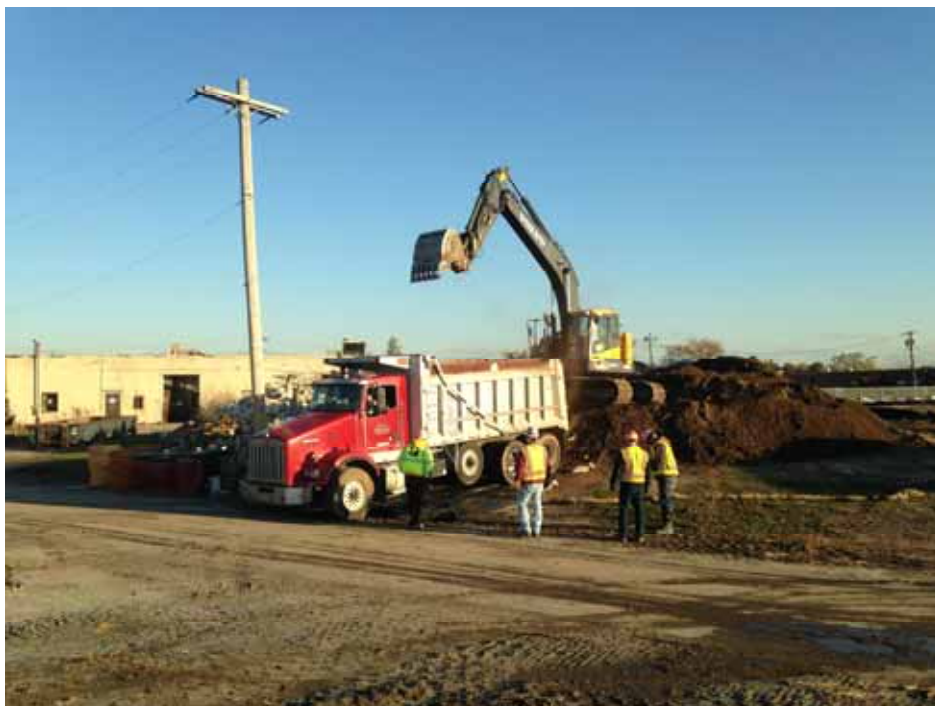
Truck being loaded with non-hazardous waste soil for offsite transportation and disposal at Gloucester County Landfill.
