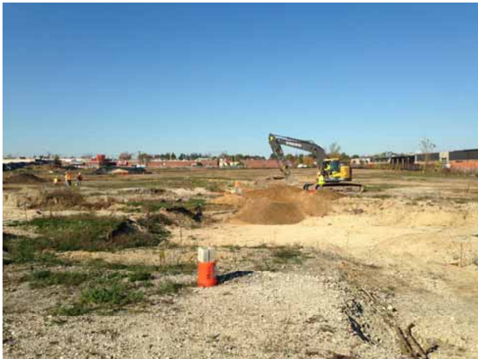
Posillico performing backfill of a leachate pit with the Volvo EC460CL Excavator.
