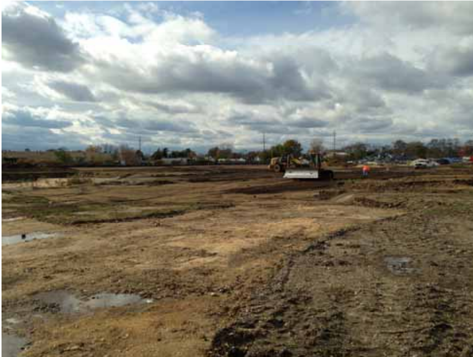
Posillico performing backfill and compaction of areas 8A, 9A, and 12B with GPS-enabled John Deere 850.
