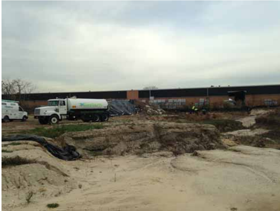
Eastern Environmental Inc. completing removal of approximately 5,000 gallons of water from the steel underground tank (suspected former tower water system return tank).
