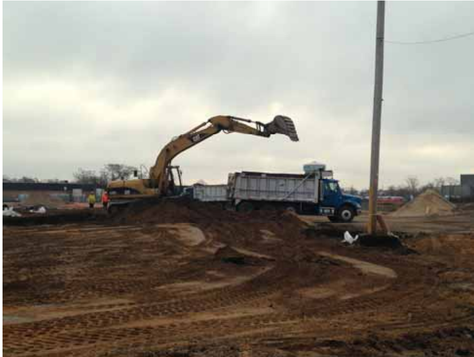
A truck being loaded with non-hazardous waste soil for offsite transportation and disposal at Gloucester County Landfill.
