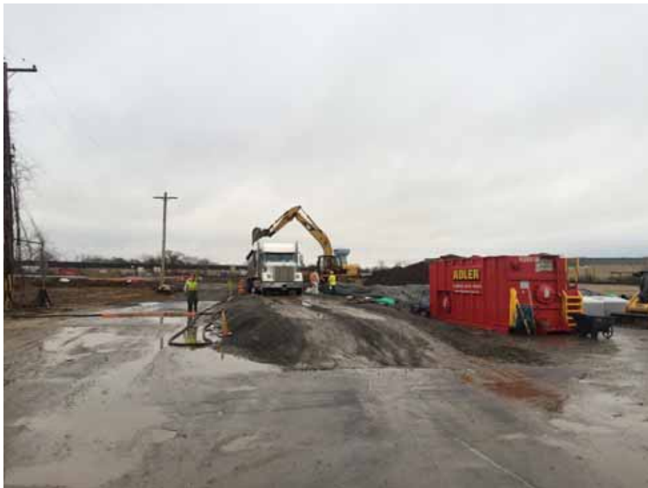
A truck being loaded with hazardous waste soil for offsite transportation and disposal at CWM Chemical Services, LLC in Model City, NY.
