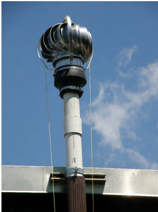
Photo 8 - Wind turbine at top of riser pipe
