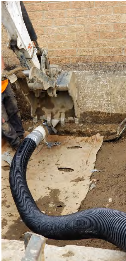
Photo 1 - Vacuum Operation at SSD-4
