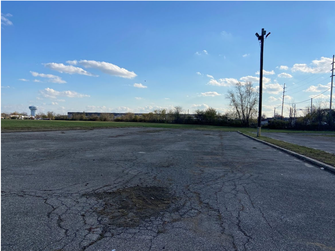
Photograph 2: Looking south, conditions of asphalt parking lot.
