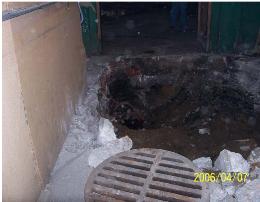
Photograph 11 - SF-07, interpreted as a storm water catch basin, was a 32-inch diameter vertical brick and concrete-walled basin with a solid bottom. The catch basin contained two 12-inch diameter terra cotta inlet/outlet pipes that were oriented generally northwest-southeast.
