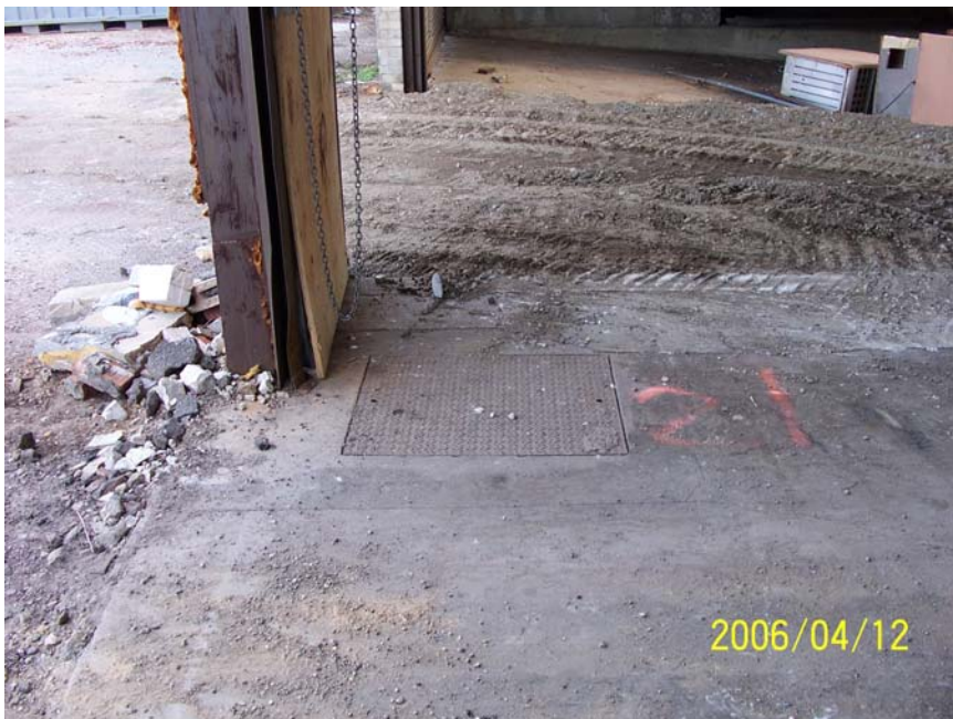
Photograph 28 – SF-21, interpreted as a former septic clean-out access sump, was a 2.5-foot square poured concrete vault with an open bottom that was covered with a steel plate.
