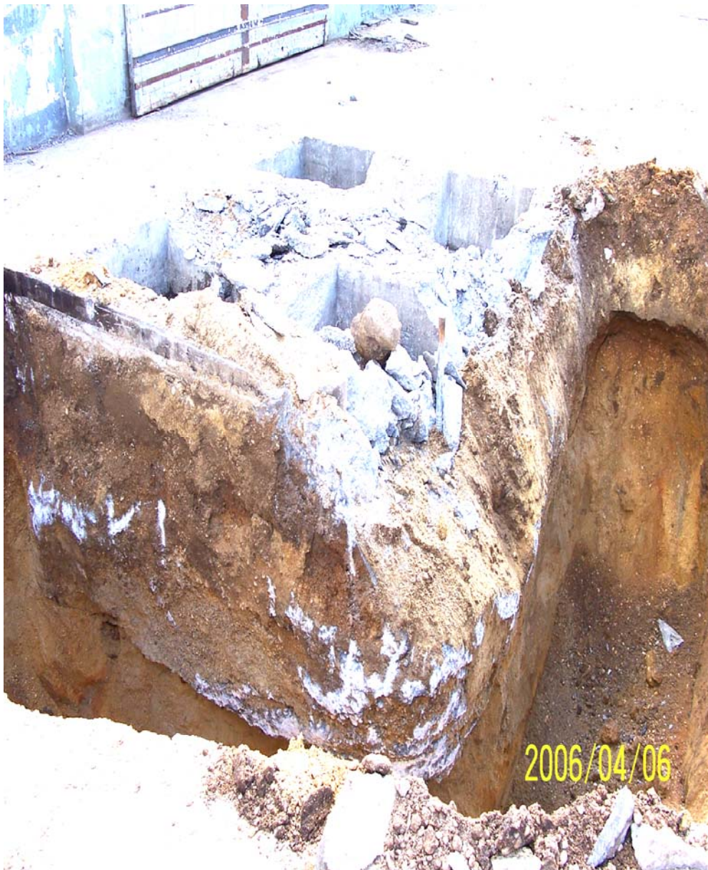
Photograph 49 – SF-47, interpreted as a former machine foundation pit, was four 2.5-foot square by 2-feet deep concrete vaults with concrete bottoms formed within a large concrete “footer.”
