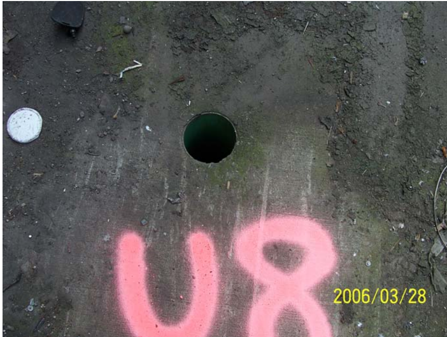
Photograph 67 – UK-08 was identified as storm water drainage pipes at the base of a loading dock within Building E. These pipes extended 2 feet vertically beneath the base of the loading dock ramp into an inaccessible vault of unknown construction.
