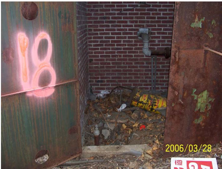
Photograph 21 - SF-18, interpreted as a former gas main access point, was a two-inch diameter vertical steel pipe. The capped steel pipe was in an enclosed seven-foot wide by seven-foot long by six-foot tall brick shed located in a courtyard east of Building A and south of Building E.
