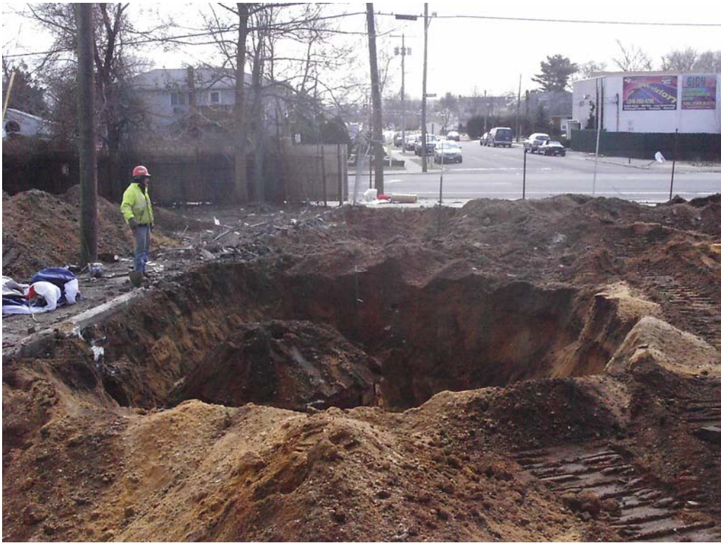
Photograph 86 – view of excavation around UK-55 (looking south) to allow evaluation prior to removal .
