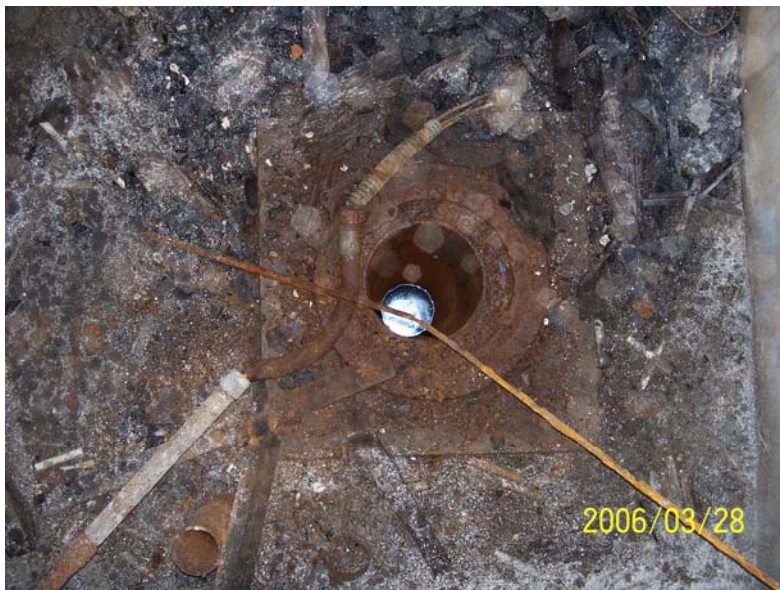
Photograph 58 – View of the 65-foot deep, 12-inch diameter water well within the SF-55 vault. The well was abandoned prior to excavation of the vault and UST.
