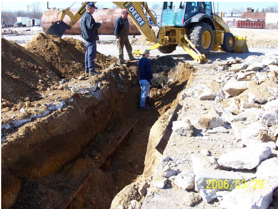
Photograph 48 – View (looking north) of SF-46 excavation and 2-inch diameter steel pipe that ran between the two vaults.
