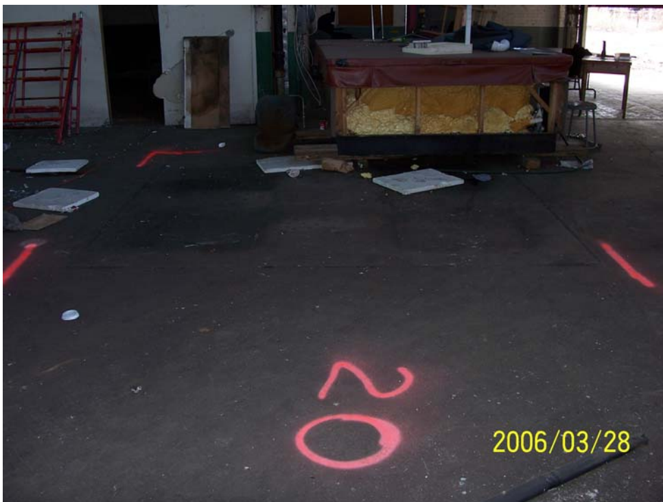
Photograph 25 – SF-20, interpreted as a former machine foundation and pit, consisted of three patched areas in the concrete floor (looking west).
