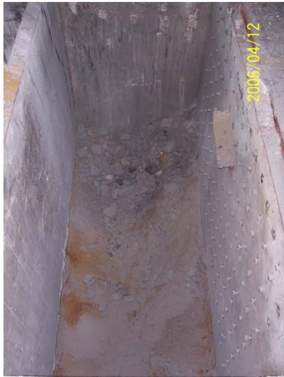
Photograph 54 – view of SF-49 vault following removal of concrete cover and demolition debris.
