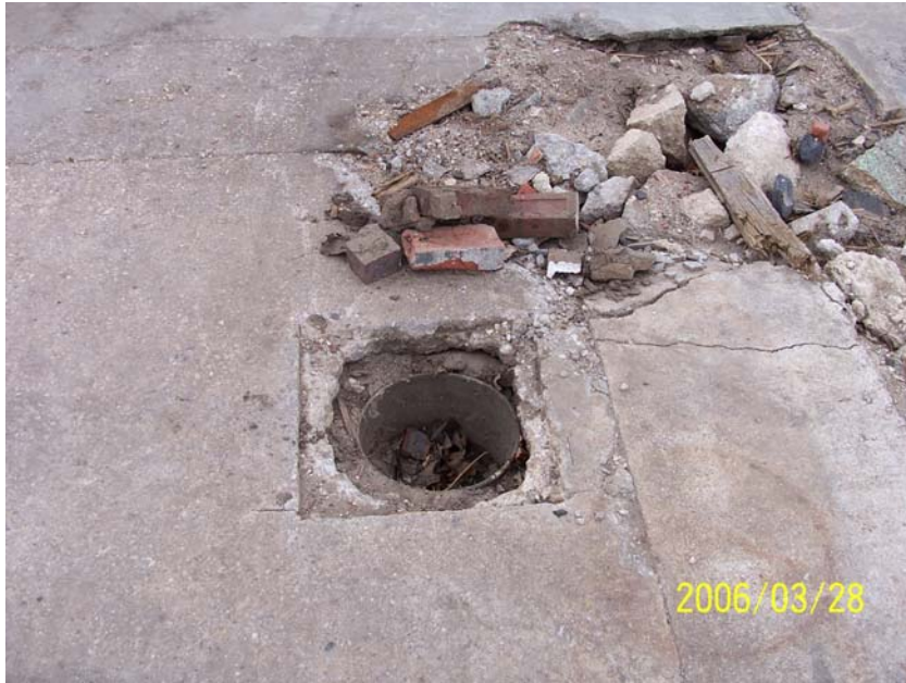
Photograph 66 - UK-07, interpreted as a blind floor sump, was a five-gallon plastic bucket placed vertically within the concrete floor of former Building A.
