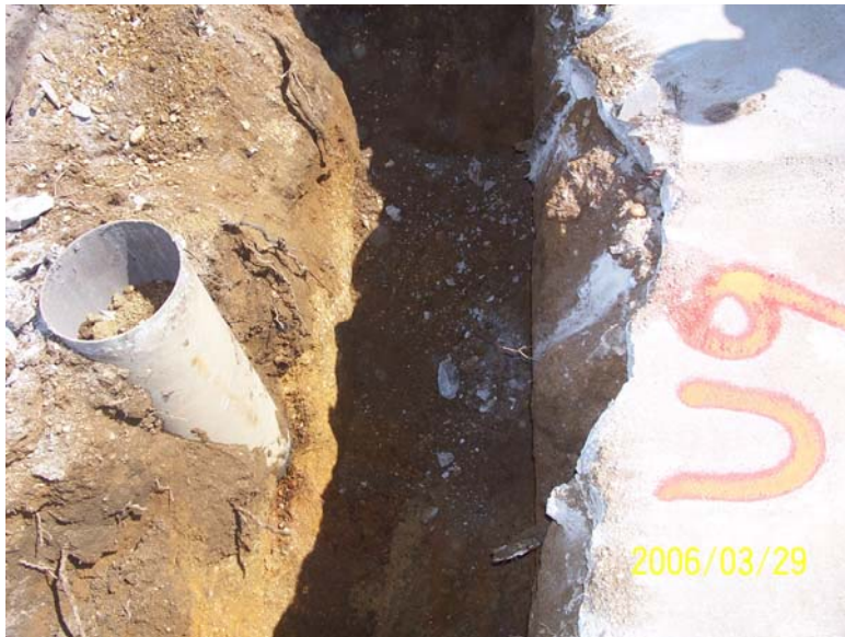
Photograph 69 - View of UK-09 during excavation. The end of cylinder was placed in sandier native material.
