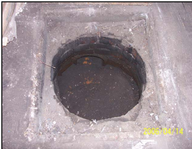
Photograph 10 - SF-06 was a 25-inch diameter vertical brick basin with a solid concrete bottom that was covered by a 37-inch square steel cover. The basin walls appeared to extend to a depth of 5-feet bgs.
