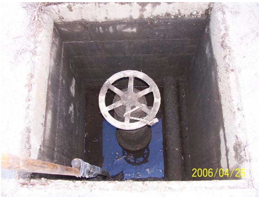
Photograph 31 – The SF-25 vault contains a 6-inch diameter steel pipe trending north-south and a vertically-oriented shut-off valve offset to the west of the pipe as shown above.
