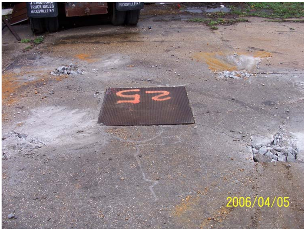
Photograph 30 – SF-25, interpreted as a fire water main access vault, was a three-foot square cinder block vault approximately four feet deep with a solid bottom and a three-foot square steel cover.
