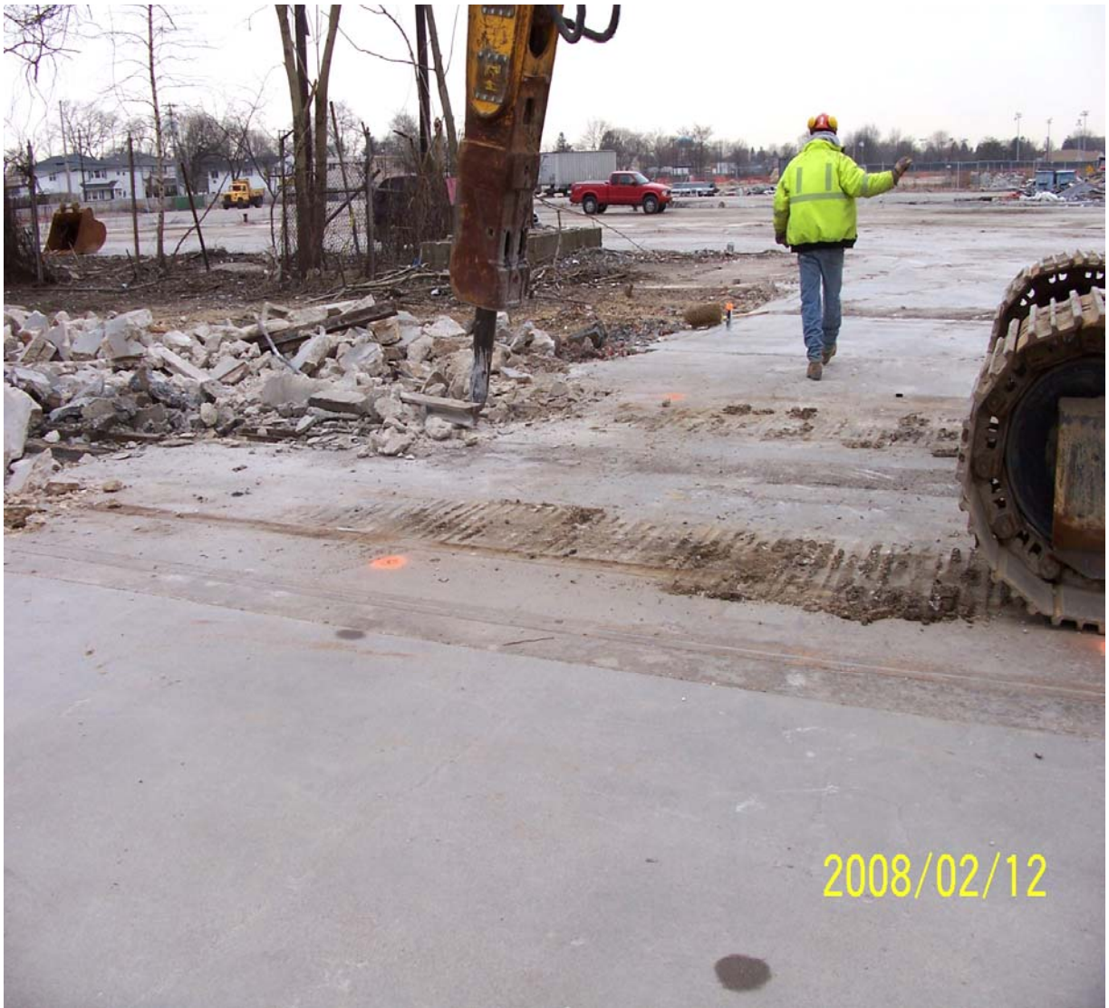
Photograph 50 – view of SF-48 during demolition. Orange painted spots near center of photograph are “fill ports”. Rail structures associated with SF-48 can be seen running from left to right (north) beneath the excavator tracks.
