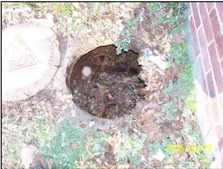
Photograph 18 – SF-15, interpreted as a former sanitary sewer access sump, was a 24-inch deep concrete basin with a solid bottom and a 20-inch diameter steel manhole cover. Three 6-inch diameter terra cotta pipes entered the basin from the west. Two pipes are plugged with wood.
