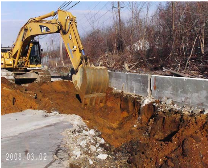
Photograph 14 - SF-08 and all associated piping was excavated and removed on March 2, 2008. The piping from SF-08 was traced to the east to UK-44, and to the west to the SF-01 excavation completed during 2006.
