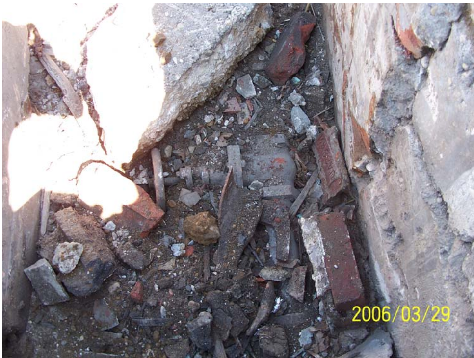
Photograph 47 – View of water supply piping and shut-off valve observed in the southern vault of SF-46.
