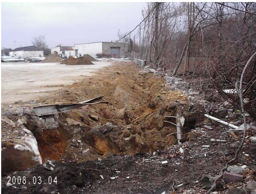
Photograph 79 – view of trench excavated to trace piping from SF-01 and SF-08 to UK-44 (looking west).
