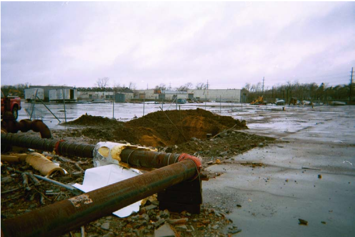
Photograph 76 – UK-42, interpreted to be a water main valve box, was located in the former pump room west of Building H (looking northwest).
