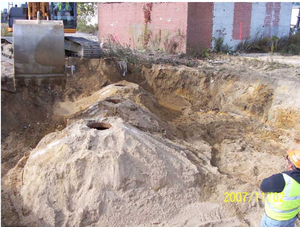
Photograph 74 – UK-37 was a series of three dry wells that were interpreted to be the southeastern most features of the Northern Leaching Chamber Field (looking northwest).
