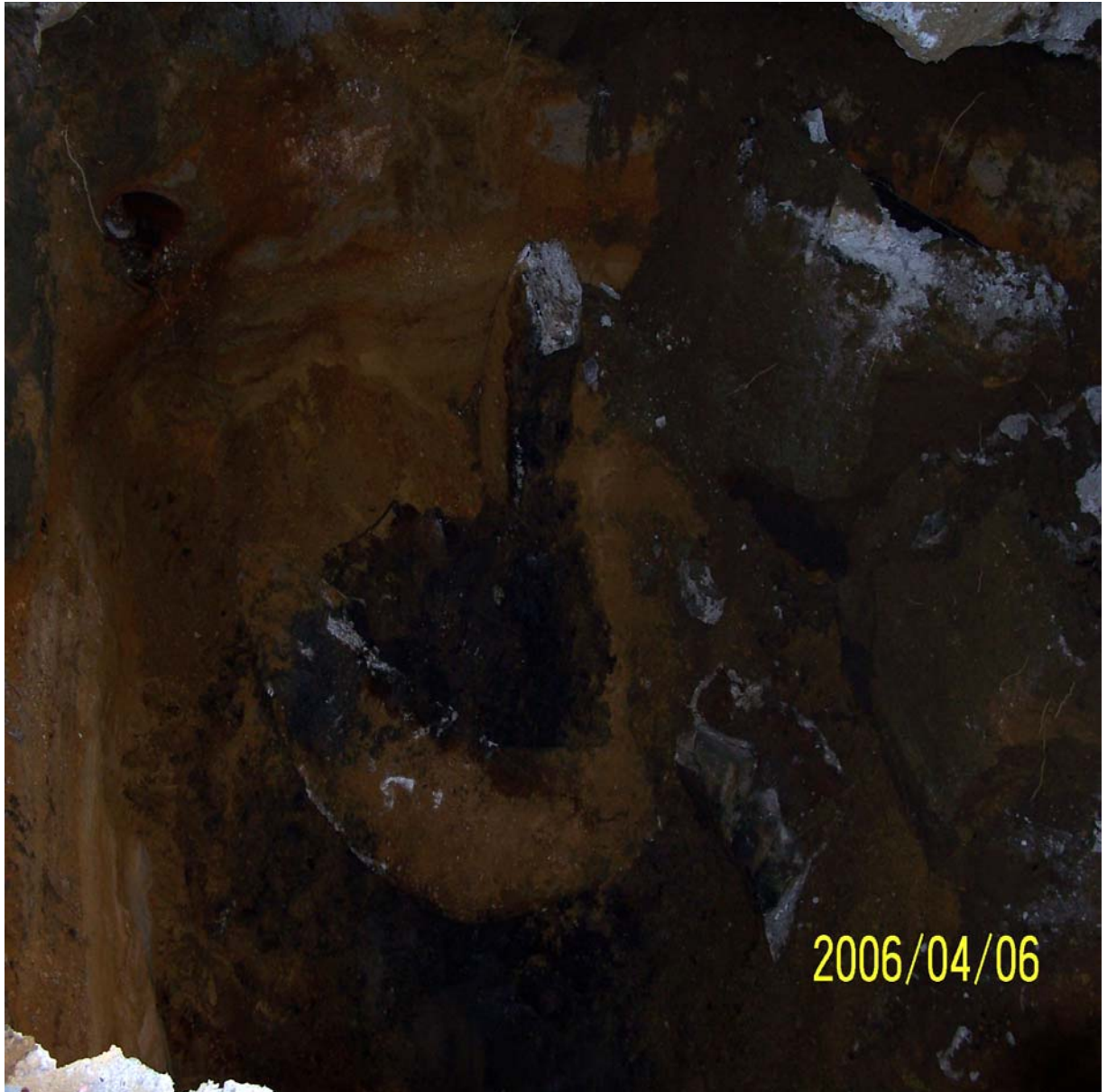
Photograph 2 – Stained soil at 12 feet bgs within SF-01. All stained soil was removed and the excavation was completed to 12.5 feet bgs.
