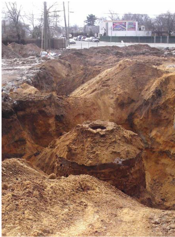
Photograph 88 – view (looking south) of excavation surrounding UK-57 to allow evaluation prior to removal.
