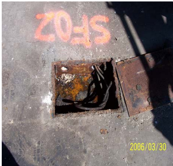
Photograph 4 – View of SF-02, interpreted as a slab-mounted utility/electrical junction box, is a 14-inch wide by 20-inch long by 8-inch deep metal box covered by a 14-inch wide by 20-inch long metal plate. SF-02 was not excavated.
