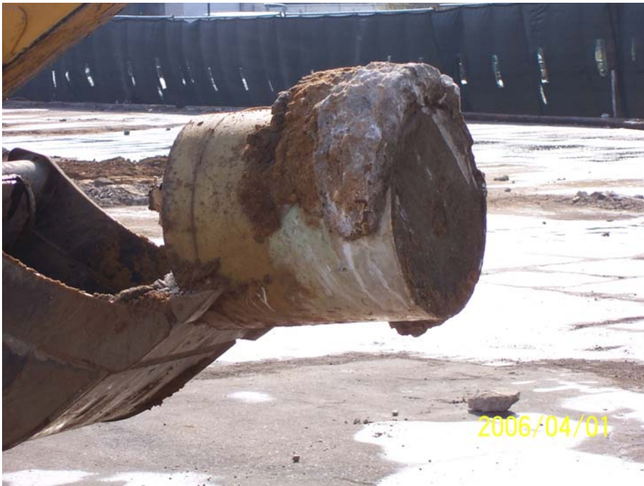
Photograph 39 - During excavation, SF-43 was identified as a vertically-oriented 19-inch diameter by 24-inch long fiberglass cylinder with an open bottom, which was filled with bentonite.
