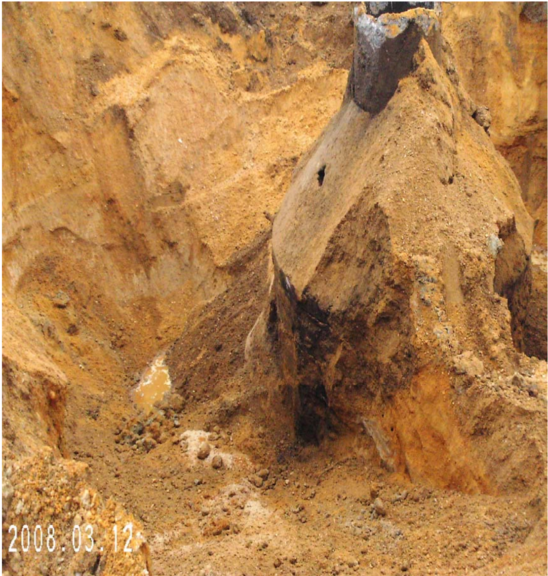
Photograph 63 – view of groundwater entering UK-01B excavation as the base of UK-01B was encountered.
