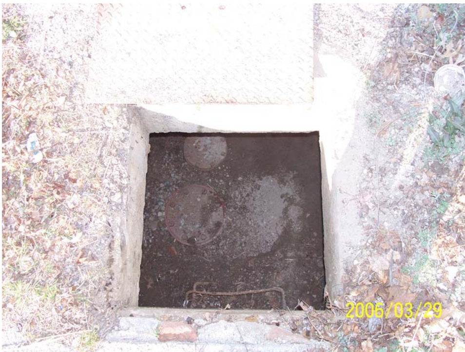
Photograph 16 – SF-14, interpreted as a city water main access vault, was a 4-foot square vault with a solid bottom approximately 5 feet deep.
