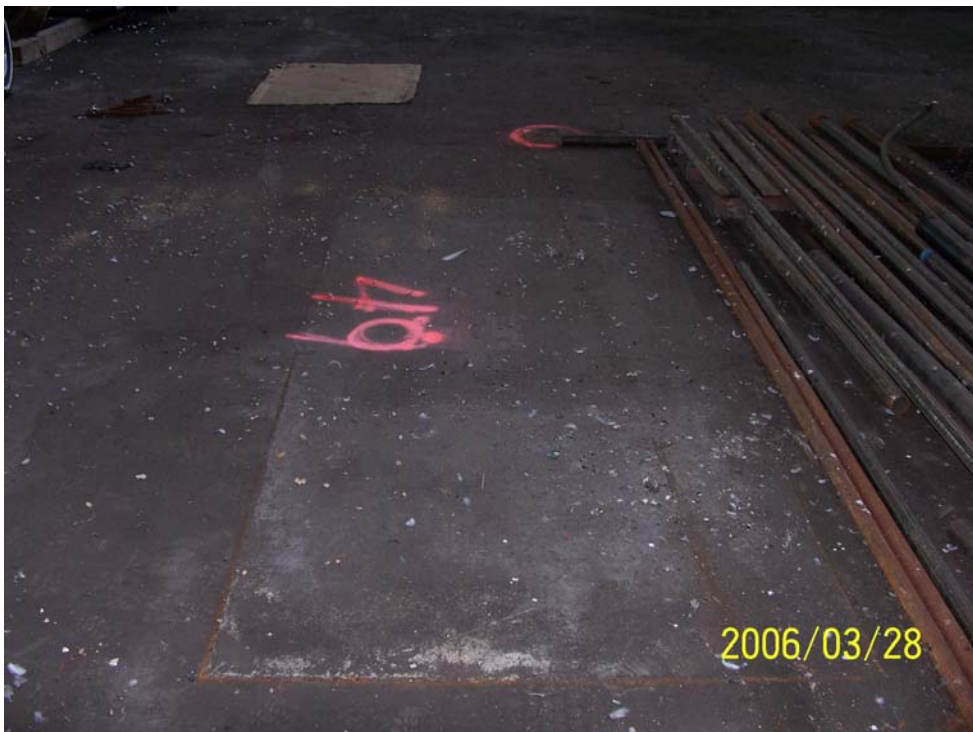
Photograph 53 – SF-49, interpreted as a former machine foundation vault, was a 4-foot wide by 9-foot long by 6-foot deep concrete vault with an open bottom that was sealed by a 4.5-foot by 9.5-foot concrete cover.
