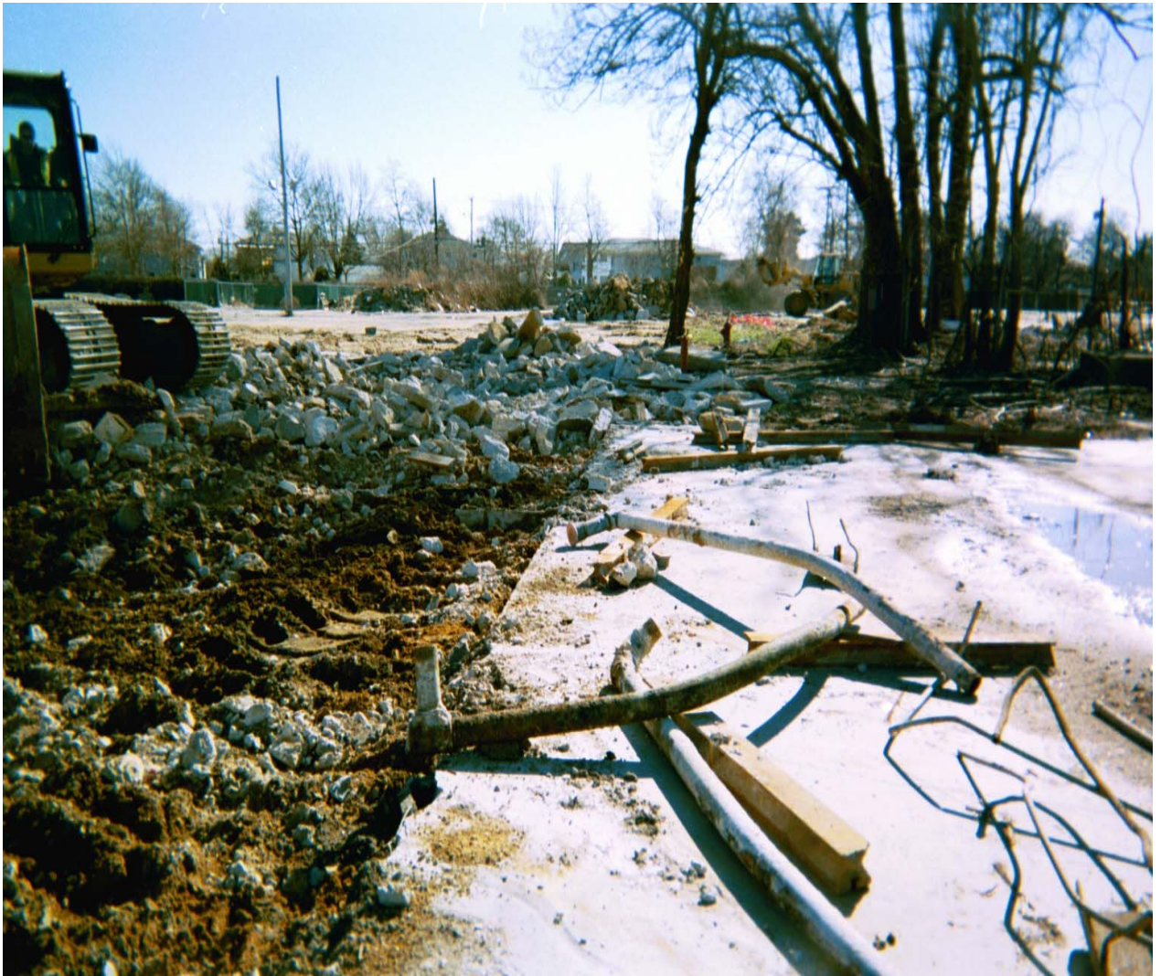
Photograph 52 – View of SF-48 during excavation showing “fill ports” and attached horizontal piping. SF-48, located within former Building U, was a series of two north-south oriented rows of fuel oil fill ports and piping, associated steel rails, and cement filled electrical boxes. Upon excavation, the fill ports and piping appeared to have been used as electrical conduits. The north and south ends of the piping entered electrical pull boxes that were also filled with cement. View is to the south.
