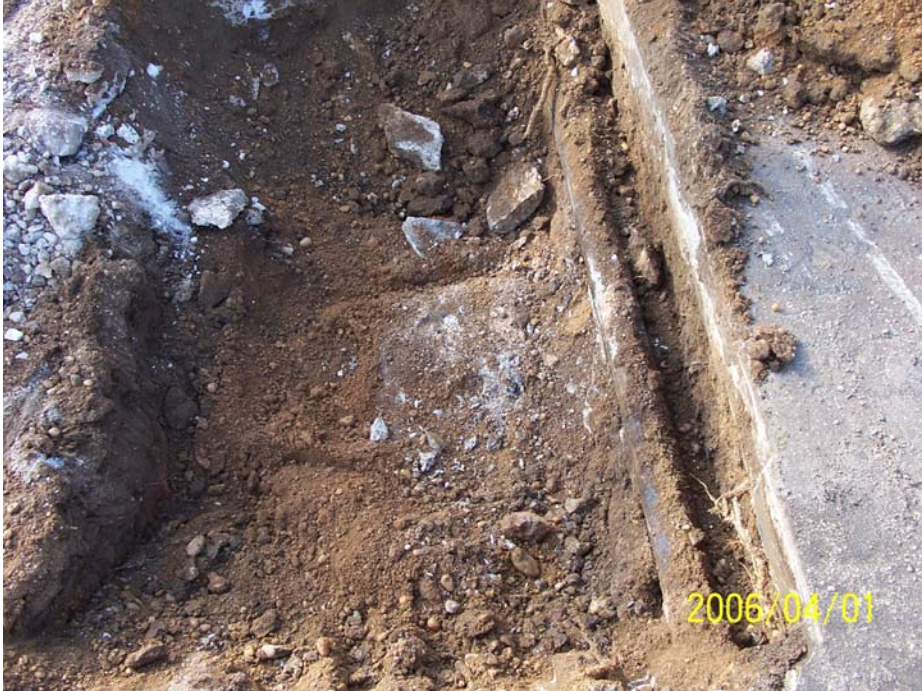
Photograph 44 - During excavation activities, SF-45 was identified as a poured concrete basin with a solid bottom. The structure contained solid resin, concrete and bentonite fill.
