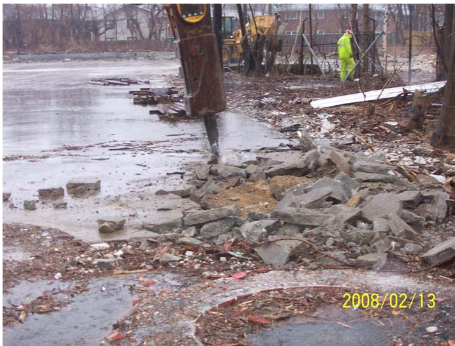
Photograph 77 – UK-43, interpreted as a former lavatory facility with sewage cleanout vaults and piping, was excavated and removed on February 13, 2008 (looking north).
