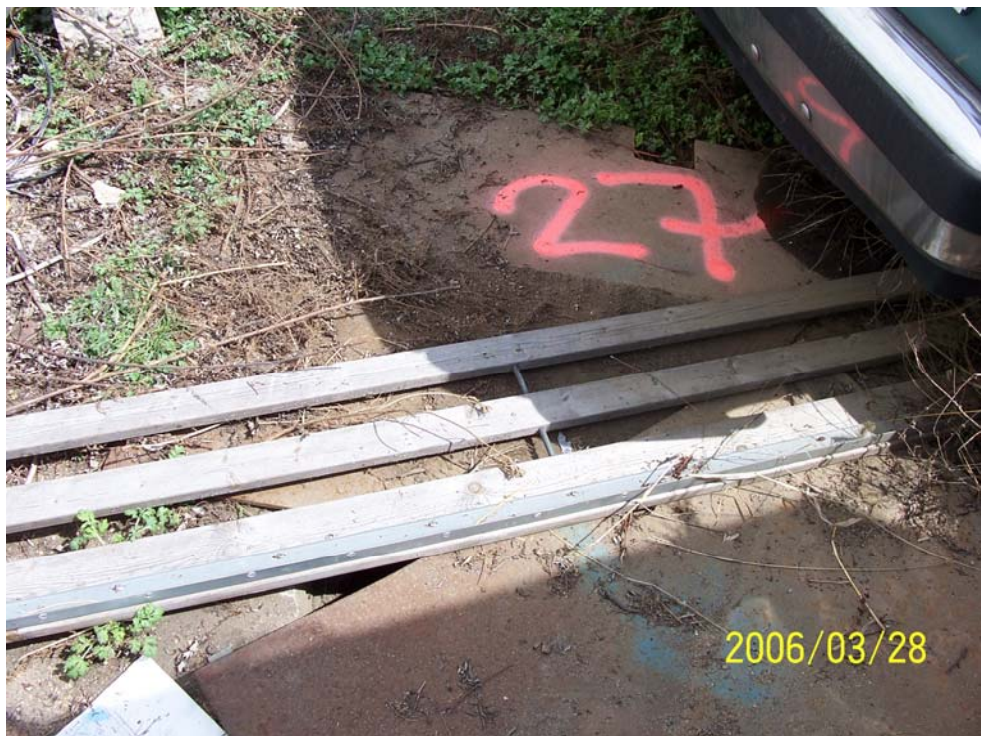
Photograph 32 - SF-27, interpreted as an electrical service access vault, was a 5-foot wide by 4-foot long by 2.5-foot deep cinder block vault that was covered by two steel plates. SF-27 had an earthen bottom.
