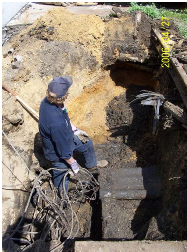
Photograph 33 - The SF-27 open-bottomed vault contained numerous electrical conduits and wires as shown above.
