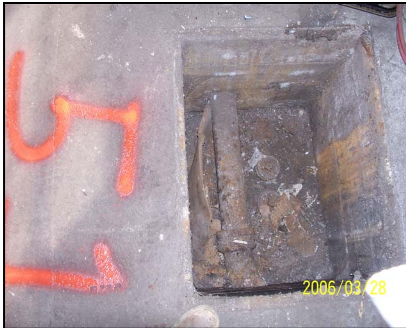
Photograph 56 – SF-51, interpreted as a former septic clean-out access vault, was a 2-foot by 2.5-foot poured concrete vault with an open bottom and covered with a metal plate. Two 4-inch diameter cast iron pipes with cleanouts were present within the vault.
