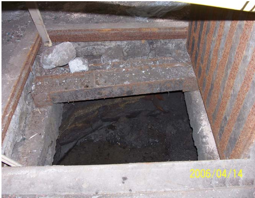
Photograph 7 - SF-04, interpreted as a storm water catch basin, was a 3-foot diameter vertical brick-walled basin, approximately 5 feet deep with an open bottom and covered by a 37-inch square steel plate.
