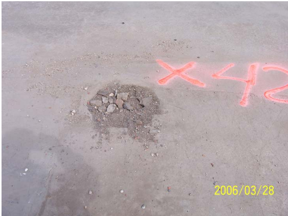
Photograph 36 - SF-42, interpreted as a blind floor sump, was a vertically-oriented 19-inch diameter by 22-inch long fiberglass cylinder with an open bottom.
