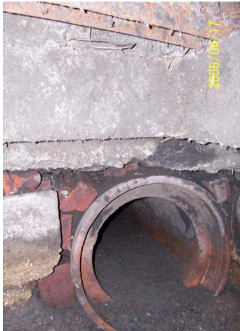
Photograph 8 - One of two horizontal 12-inch diameter terra cotta inlet/outlet pipes located at ~3 feet bgs within SF-04.
