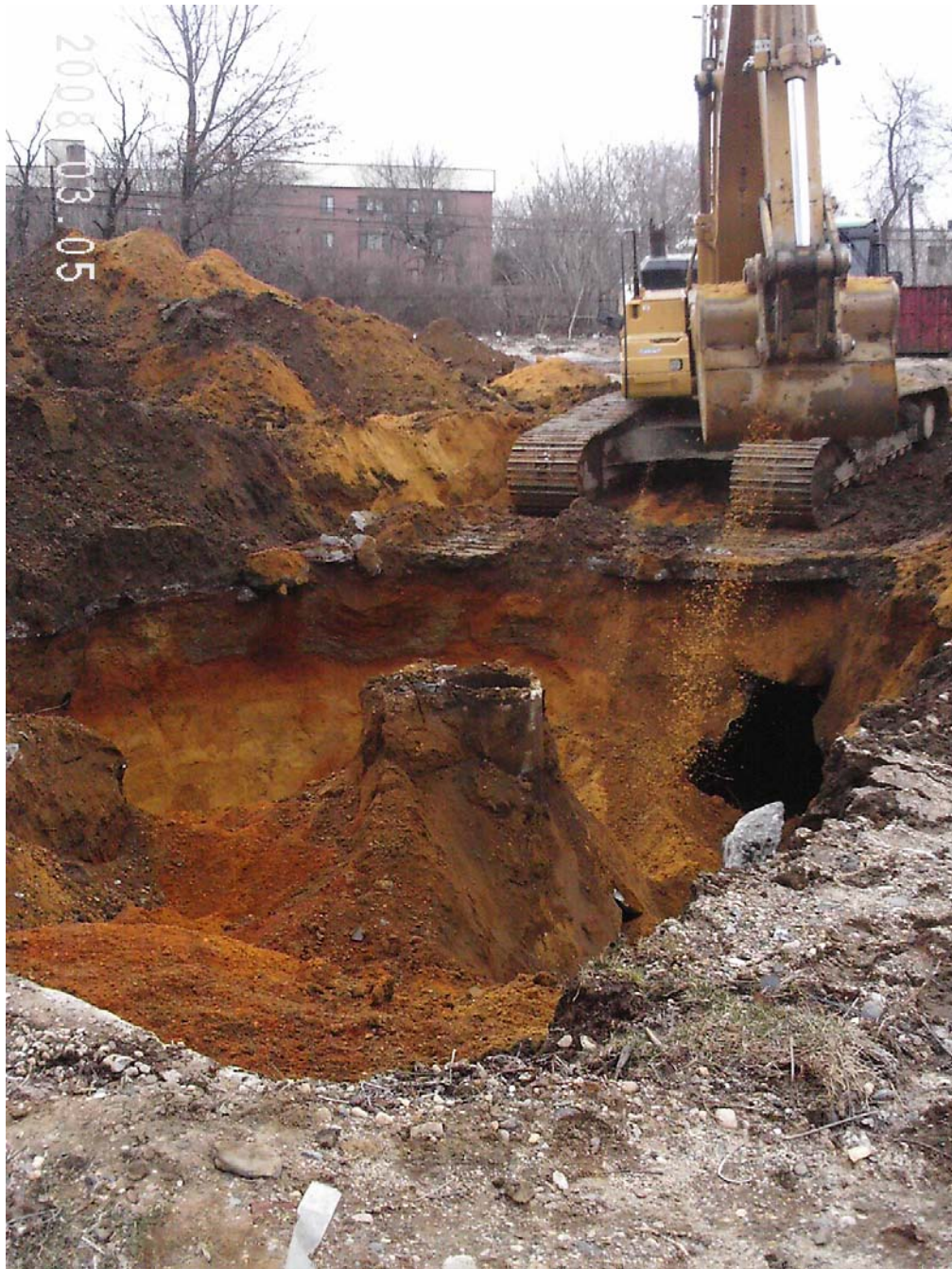
Photograph 61 – Upon excavation, piping from UK-01 was traced to this dry well located south of UK-01. Piping from this drywell was traced east to UK-01A. The broken sidewall of UK-01A can be seen at the right of the photograph beneath the excavator. View is to the northeast.
