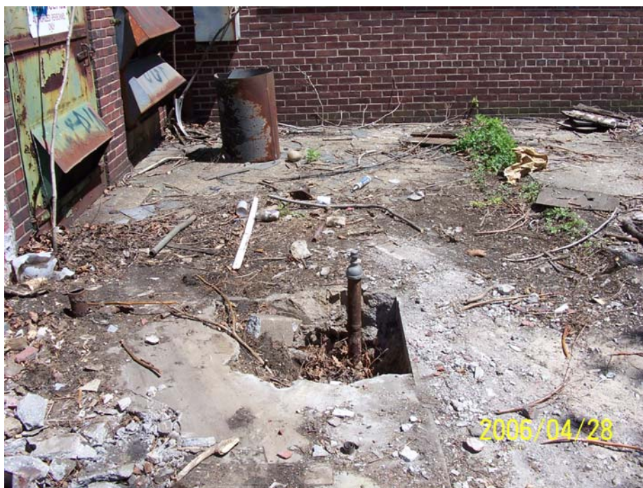
Photograph 22 – View of SF-18 gas main pipe following demolition of the brick enclosure (looking east).
