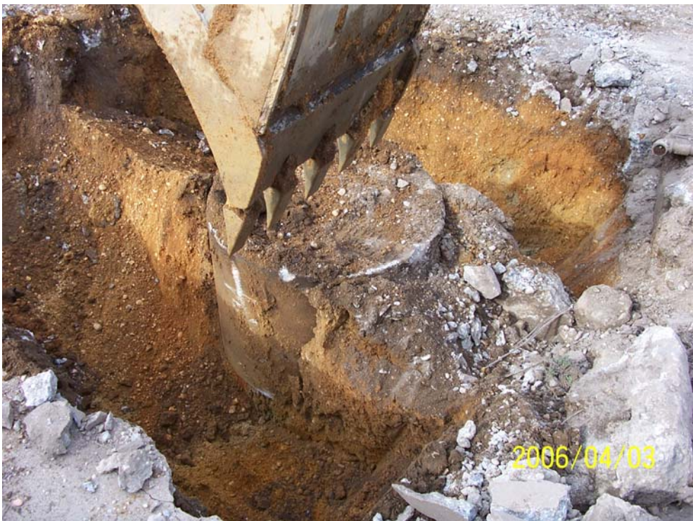
Photograph 70 – UK-10, interpreted as a blind floor sump, was a 32-inch diameter concrete basin with a concrete bottom covered by a 24-inch diameter metal drainage grate.
