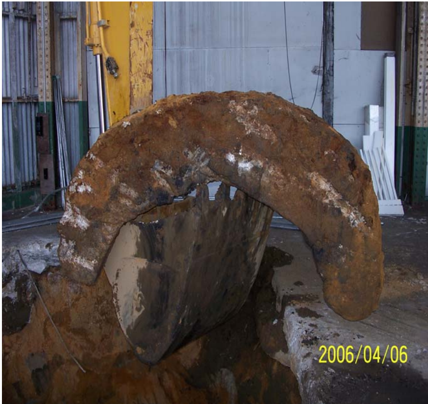
Photograph 3 – Portion of an 8-foot diameter, 1-foot thick by 1-foot wide concrete ring that was encountered at a depth of 11.5 feet bgs within SF-01.
