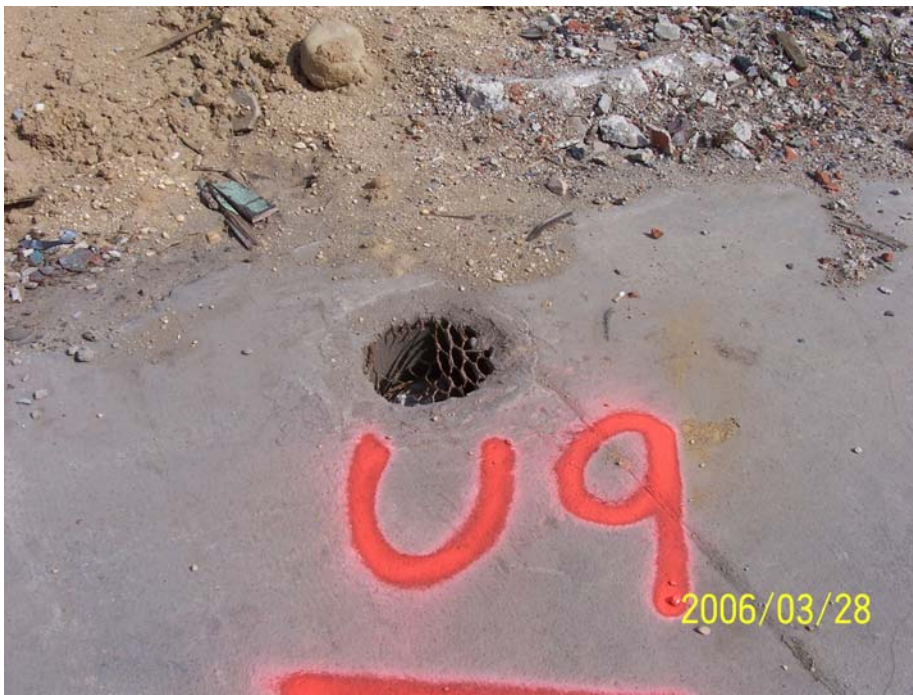
Photograph 68 – UK-09, identified as a blind floor sump, was a 12-inch diameter by 38-inch long open-bottomed fiberglass pipe with an expanded metal screen at the top.
