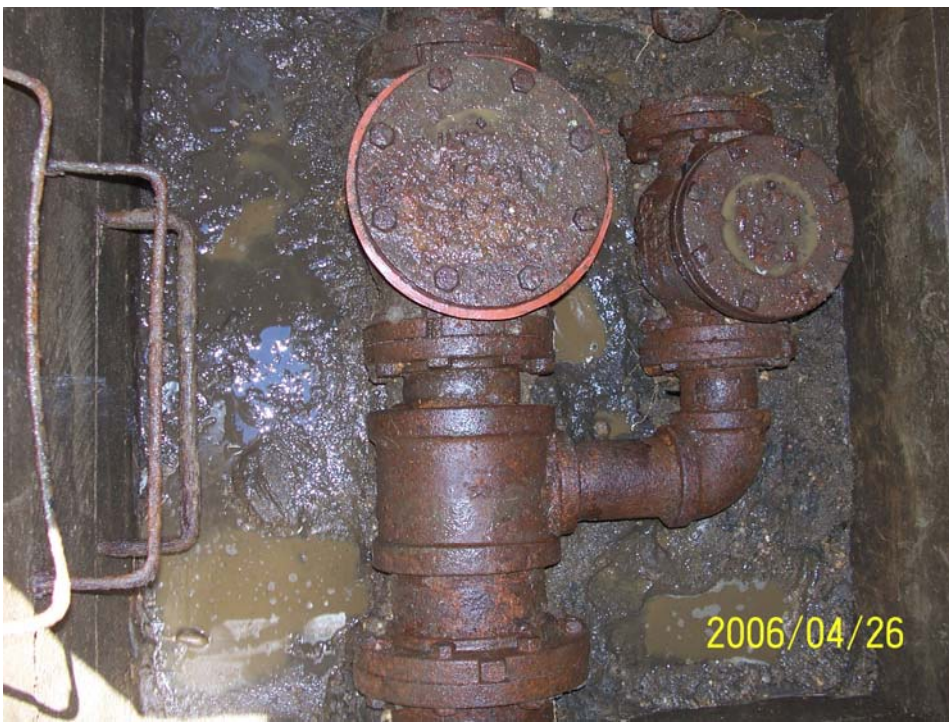
Photograph 17 – View of a 10-inch diameter water main with two capped valve boxes trending north-south within the SF-14 vault.
