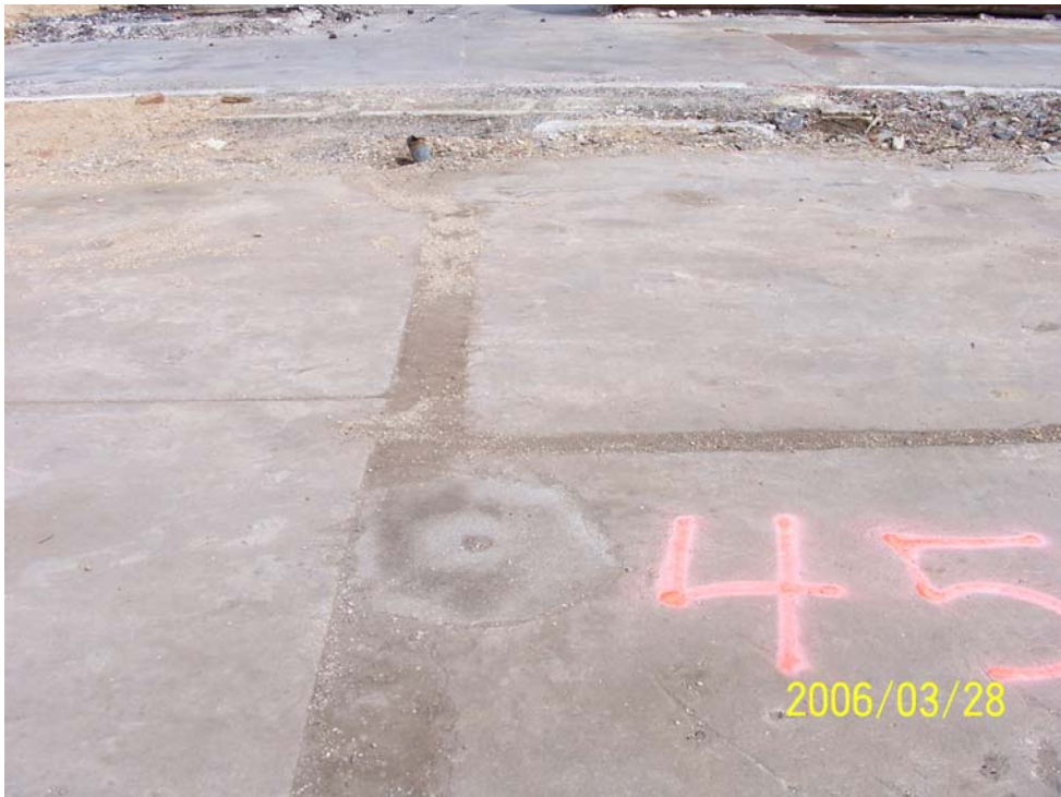
Photograph 43 – SF-45, interpreted as a blind floor sump, was initially identified as a two-foot diameter depression and concrete patch in the floor slab of former Building A as shown above.
