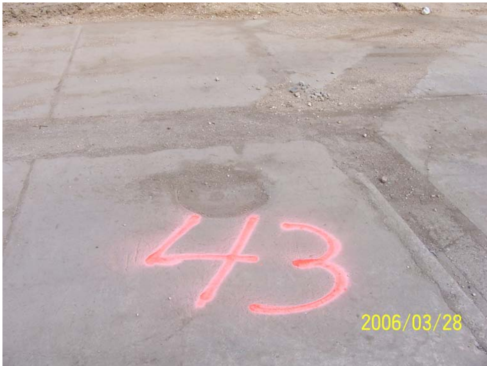
Photograph 38 - SF-43, interpreted as a blind floor sump, was initially identified as an 18-inch diameter circular depression in the concrete floor slab of former Building A as shown above.
