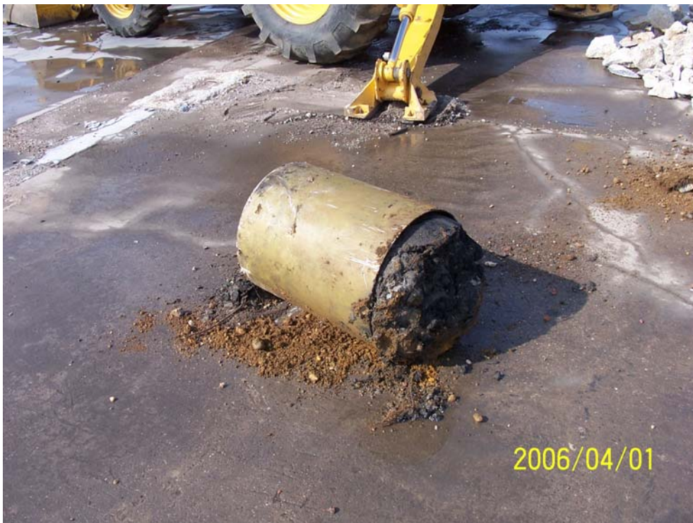
Photograph 37 – The open-bottomed fiberglass cylinder at SF-42 was filled with sediment, concrete and brick debris.
