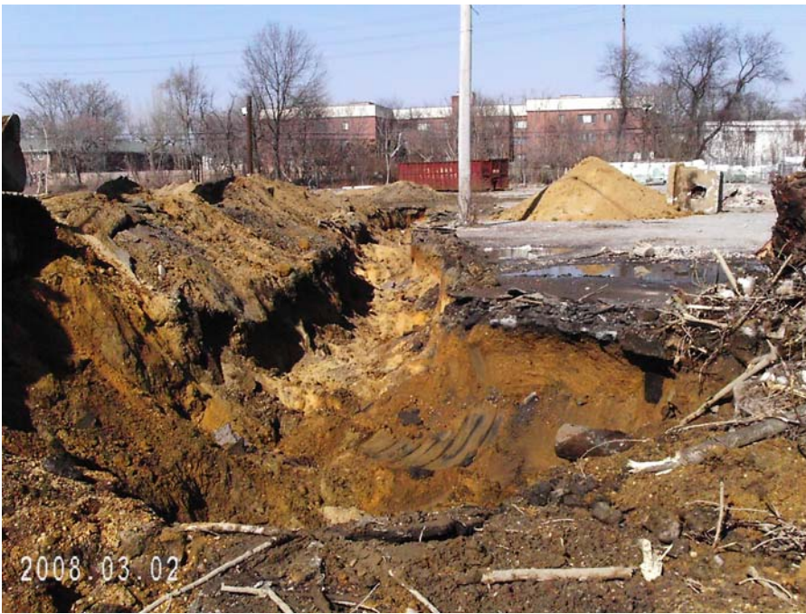
Photograph 90 – view of pipe excavation from UK-45, which led to the discovery of UK-59. Pipe that exited UK-59 can be seen at the lower right of the photo.
