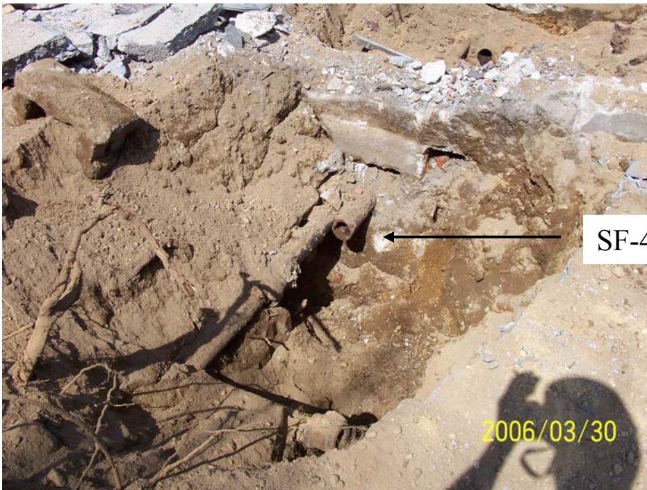
Photograph 42 – The SF-44 floor drain was a 3-inch diameter vertical steel drain pipe located inside a 9-foot by 15-foot concrete structure. The pipe discharged to a small 4-foot square by 2-foot deep cinder block vault with an earthen bottom.
