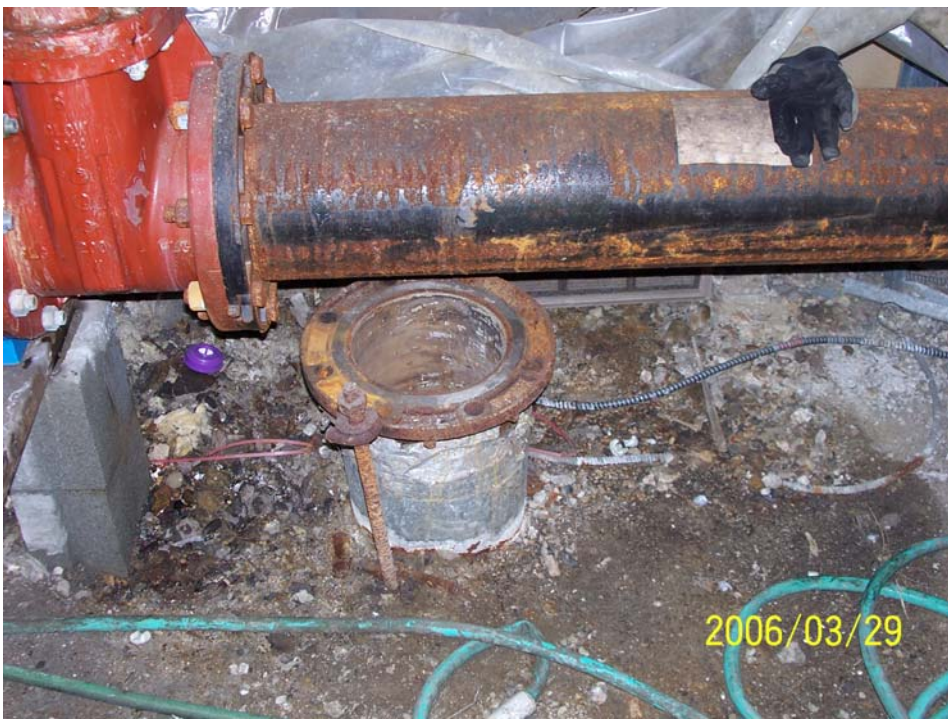
Photograph 15 - SF-13, interpreted as a fire water main access vault, was historically identified as a 2-foot by 3-foot cinder block structure with a steel cover. The only subsurface feature AMO observed in the vicinity of SF-13 was an 8-inch diameter steel pipe shown above.
