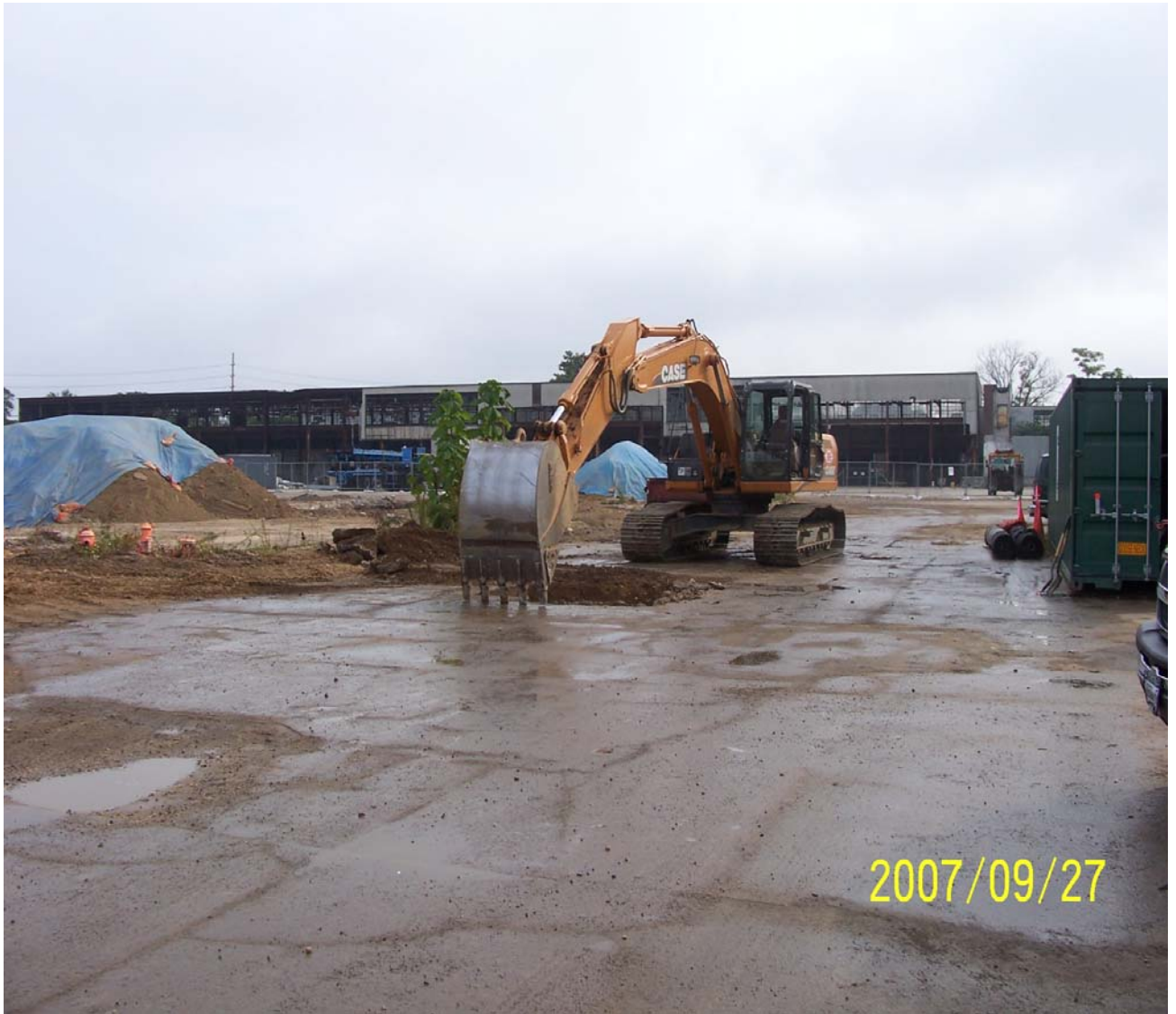
Photograph 72 – UK-33/UST-13 vault was located within the former Building A slab (view to the east).
