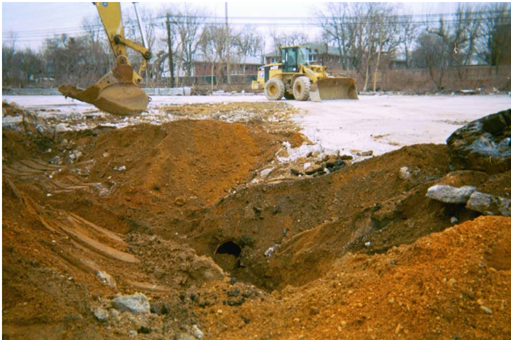
Photograph 83 – view of UK-46 excavation and pipe running to the north (looking north). Pipe was traced to the north where it intersected with pipe connecting SF-01, SF-08 and UK-44.
