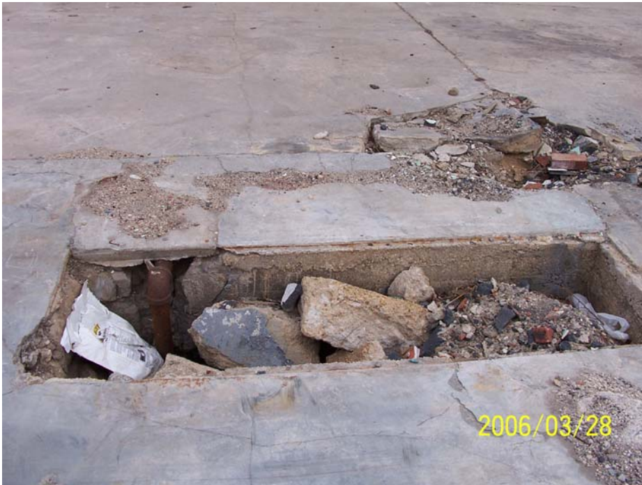
Photograph 46 – View above is of a 2.0-foot by 4.0-foot vault. The vault contained a vertical steel pipe that connected to the vault located approximately 23 feet to the north. Vault was filled with sediment, brick and concrete debris.
