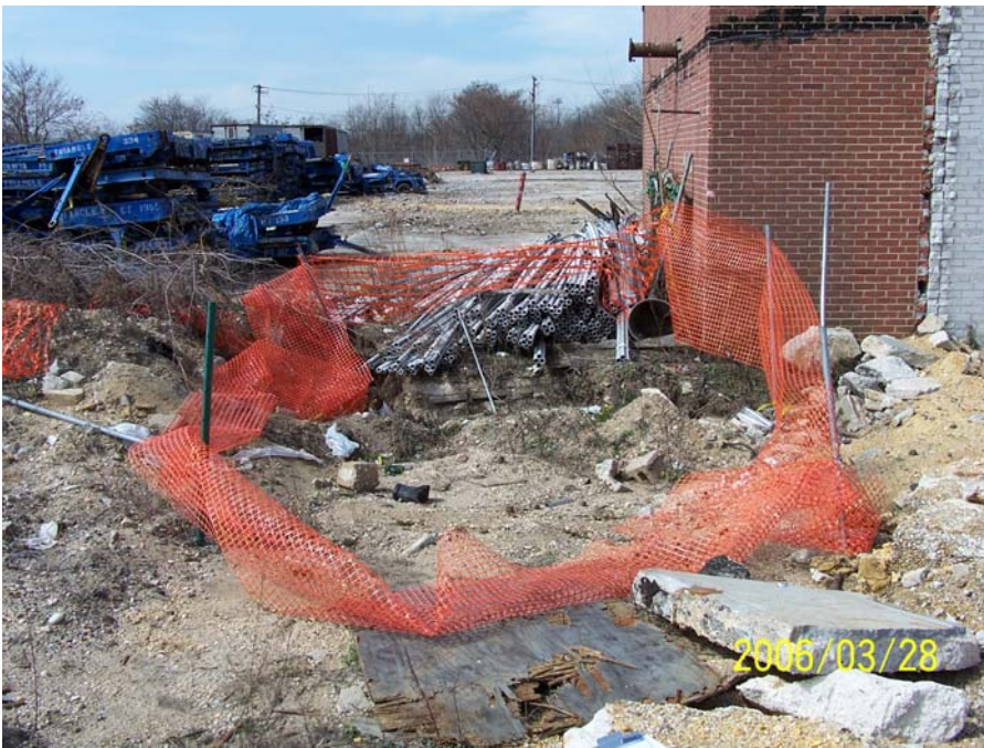
Photograph 64 - UK-05, interpreted as potentially being associated with the Northern Leaching Chamber Field, was visible as a depression partially beneath an 18-inch thick concrete slab south of the “small brick building” (looking west).
