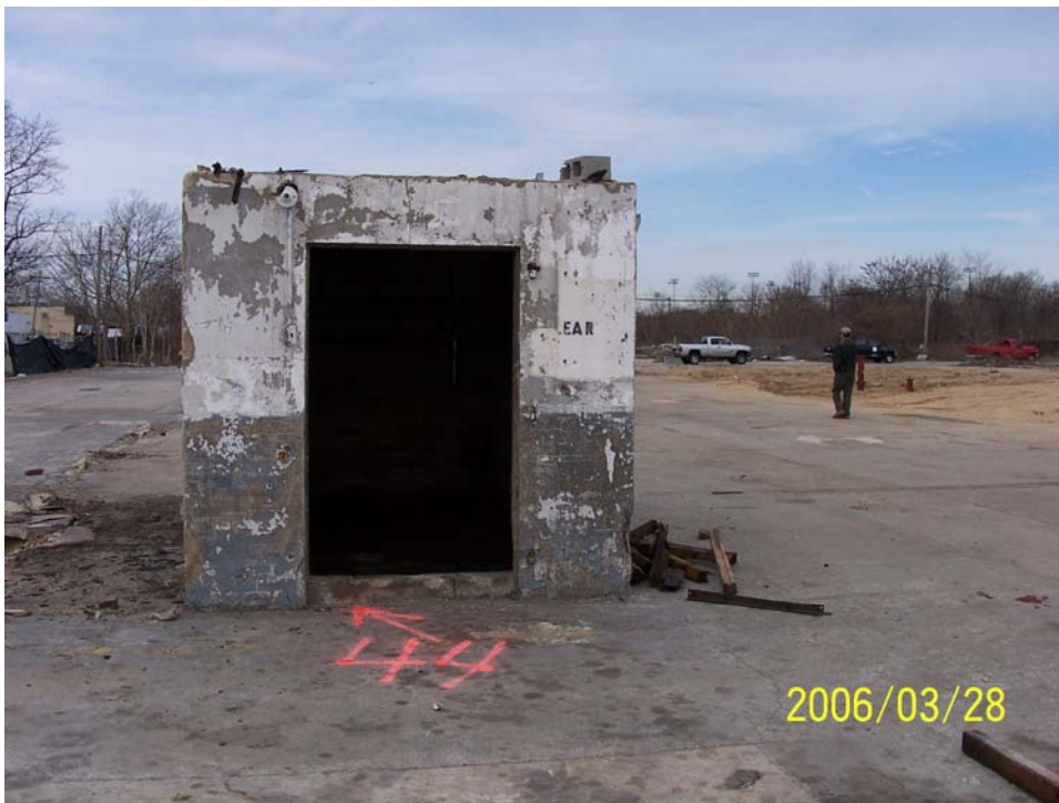
Photograph 41 - SF-44, interpreted as a floor drain in a former electrical room, was located within former Building A.
