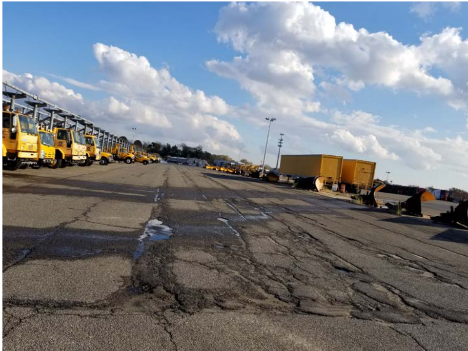
Asphalt Surface Cracks Area C
