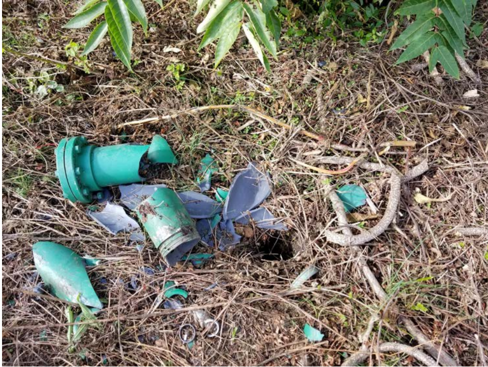
Well Casing Broken at Grade – NW-3
