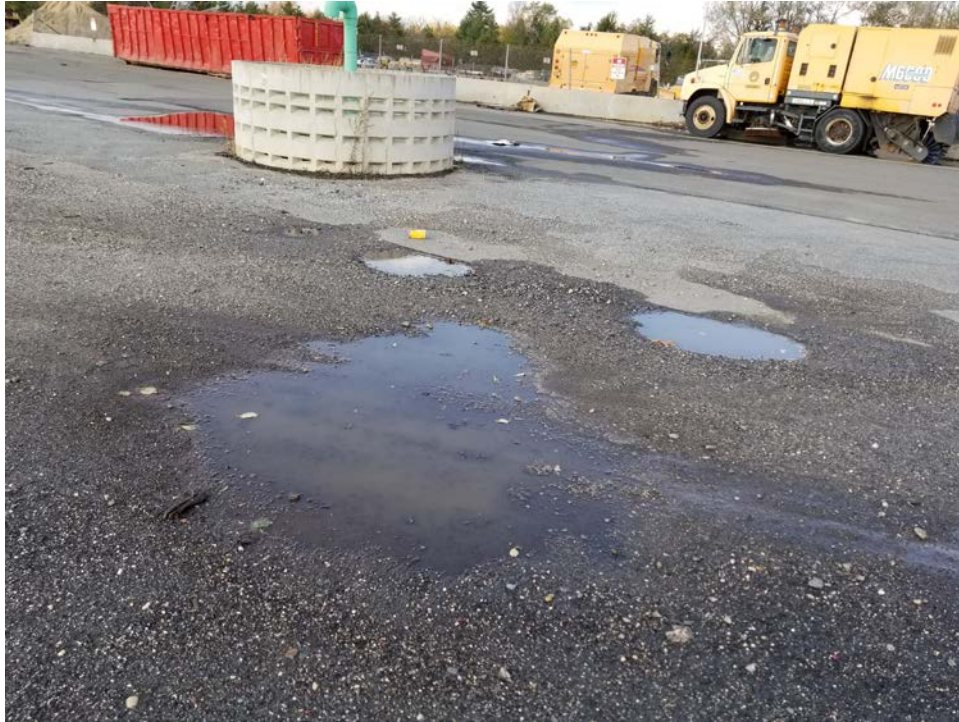
Ponding in Area A/C Border
