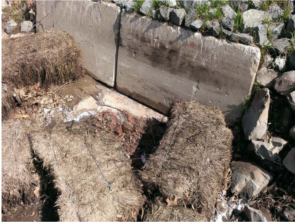
Siltation – Catch Basin #5
