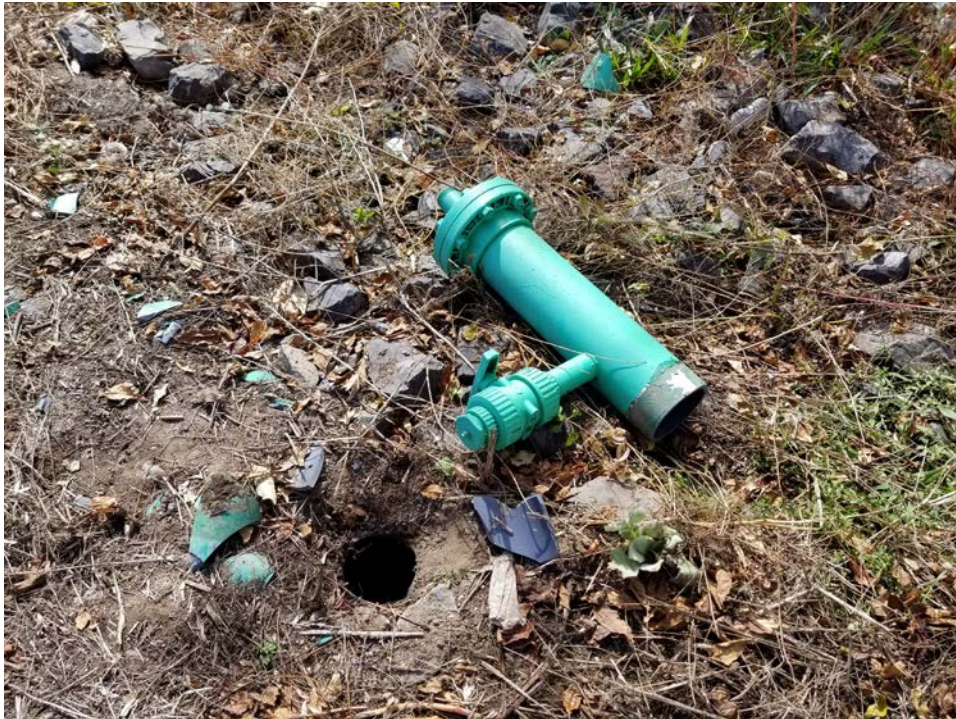
Well Casing Broken at Grade – SW-6
