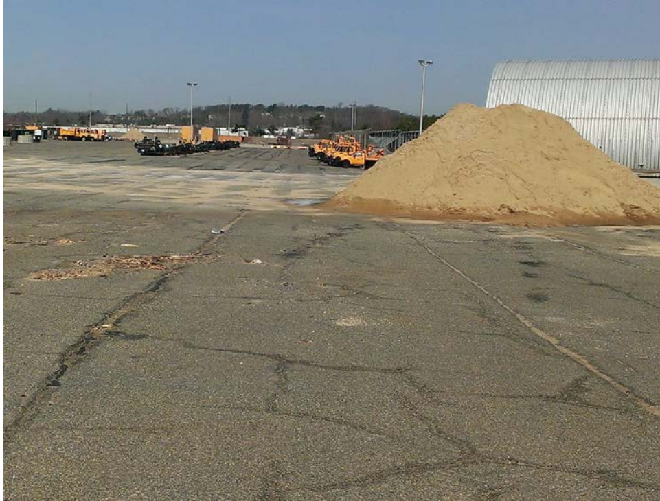
Asphalt Surface Cracks in in Area C
