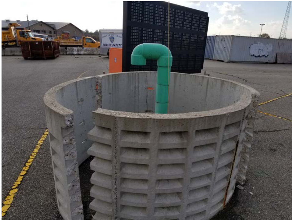
Ridge Gas Vent Well Broken Ring – R-26
