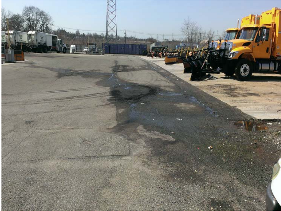
Minor Ponding in Area E
