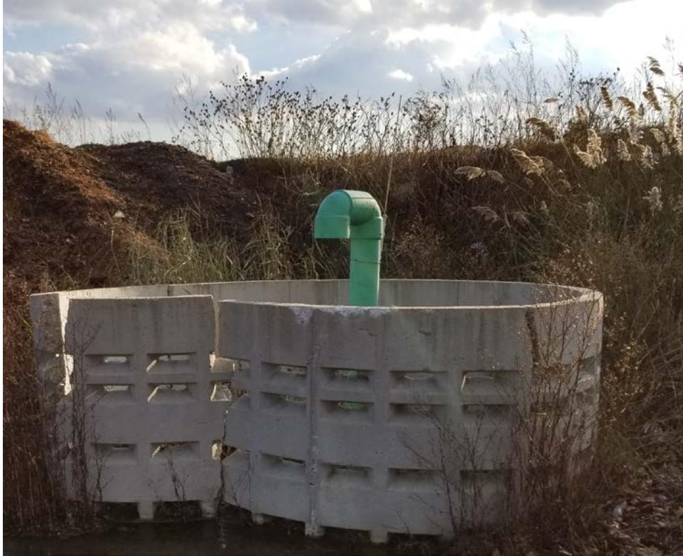
Ridge Gas Vent Well Broken Ring – R-6
