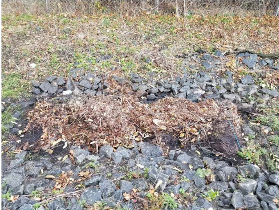
Siltation/Debris – Catch Basin #2
