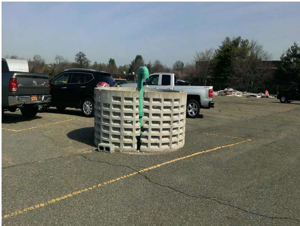
Ridge Gas Vent Well Broken Ring – R-26
