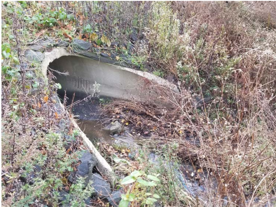
Some Siltation and Vegetative Growth – ES#1 (DS#8)
