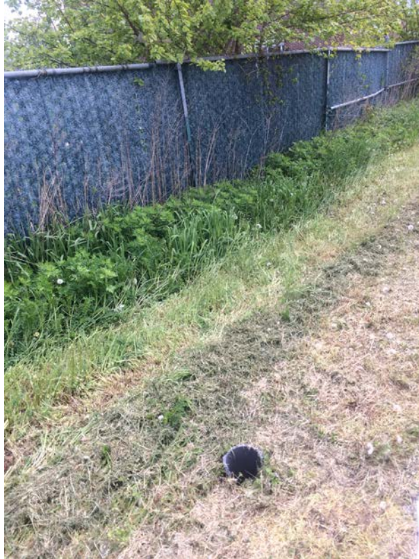
Well Casing Broken at Grade – NE-16
