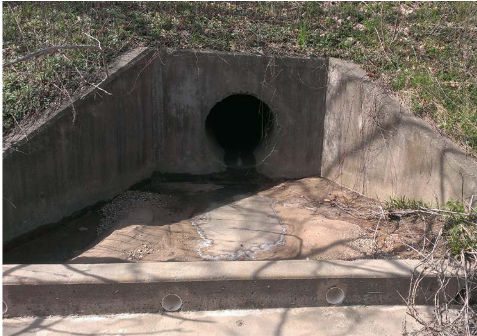
Minor Siltation – RB #284 (HW #3)
