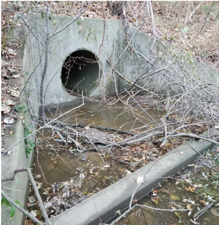
Minor Siltation/Debris – RB #358 (HW #4)
