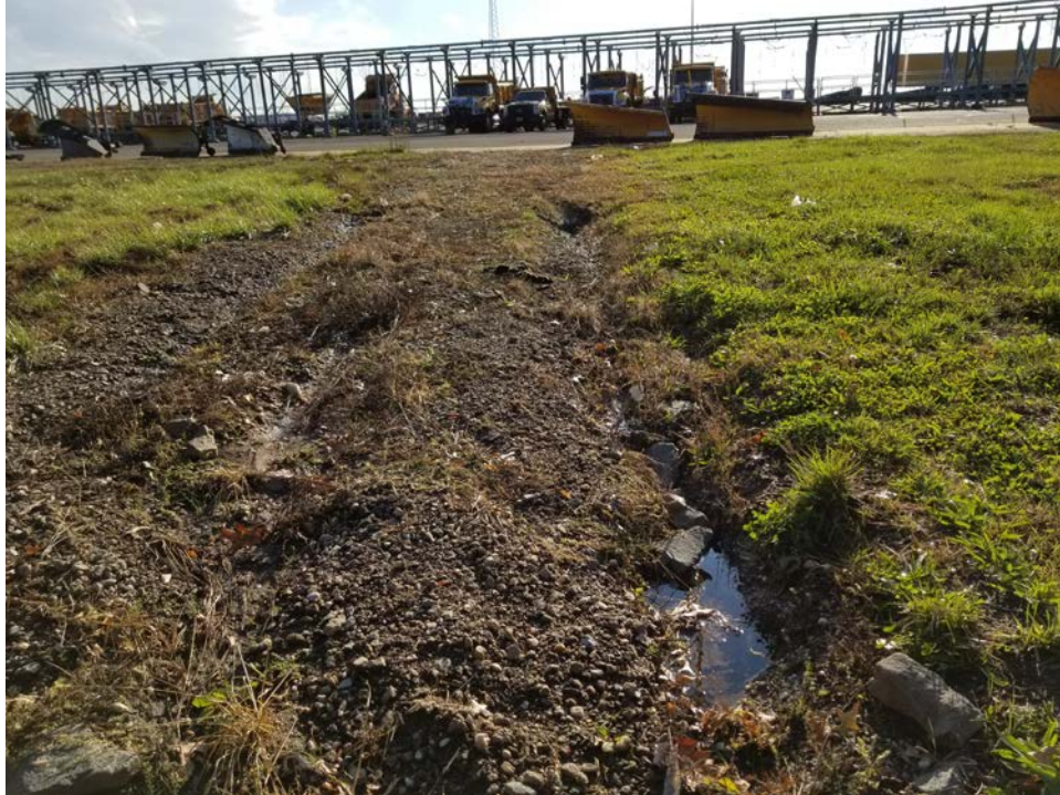
Vegetative Cover Erosion in Area C
