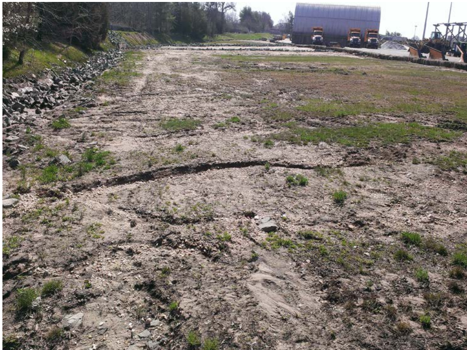
Surface Material Erosion in Area C
