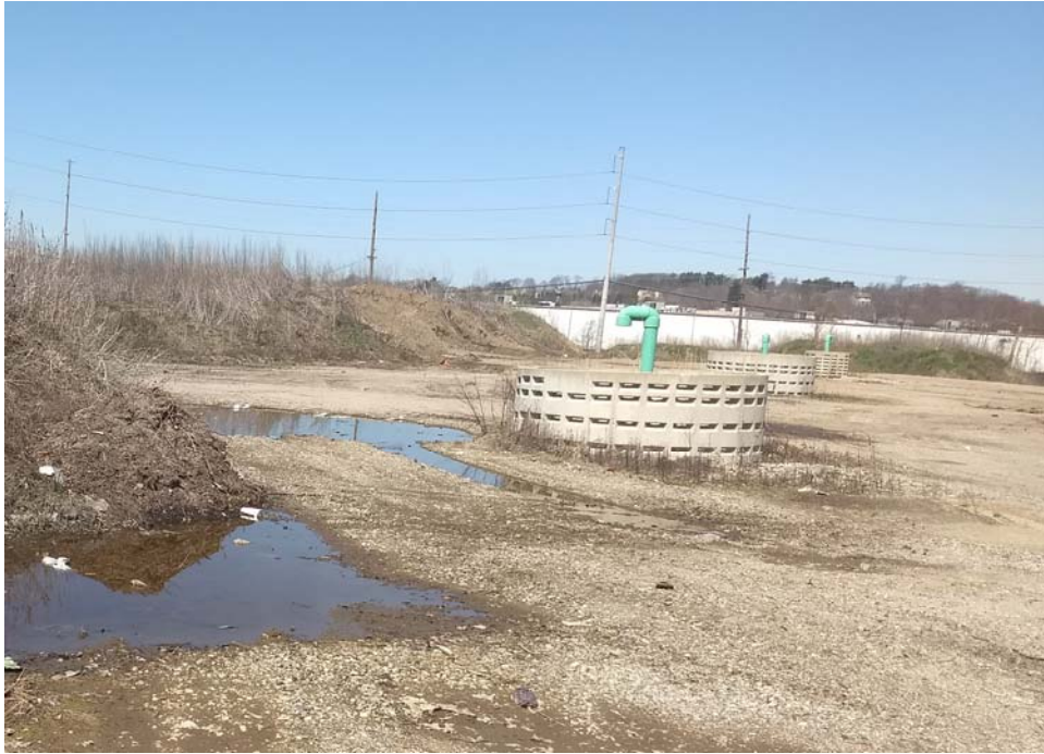
Minor Ponding in Area A
