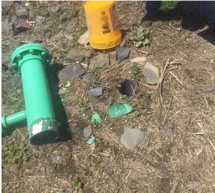
Well Broken at Grade – SW-6
