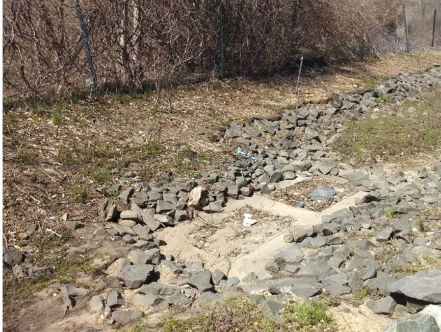
Siltation and debris – Catch Basin #2
