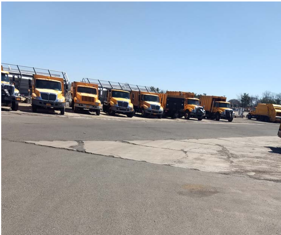
Minor surface cracks in Area E
