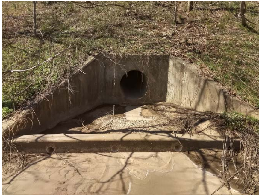
Minor Siltation – RB#284
