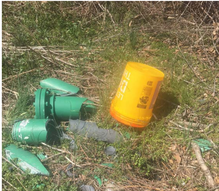
Well Broken at Grade – NW-3
