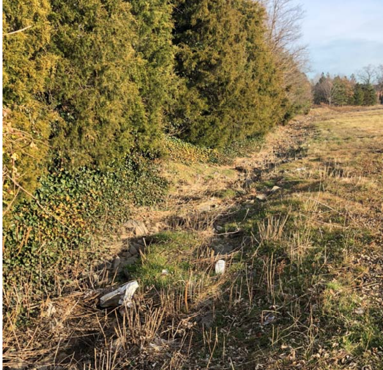
Siltation, vegetative growth and debris- DS#3
