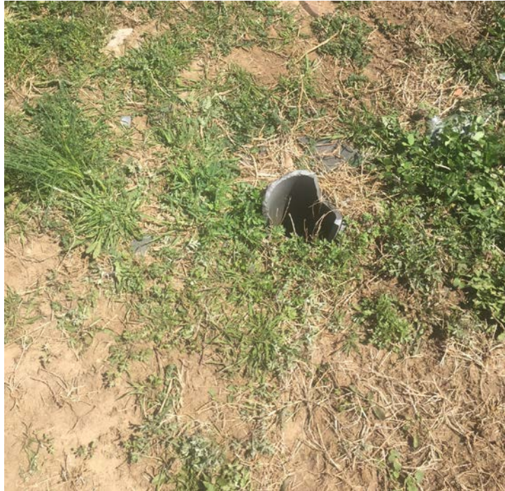
Well Broken at Grade – NE-16
