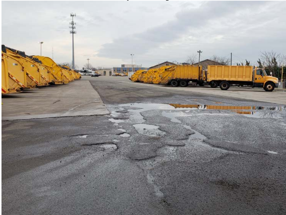
Minor Ponding in Area E
