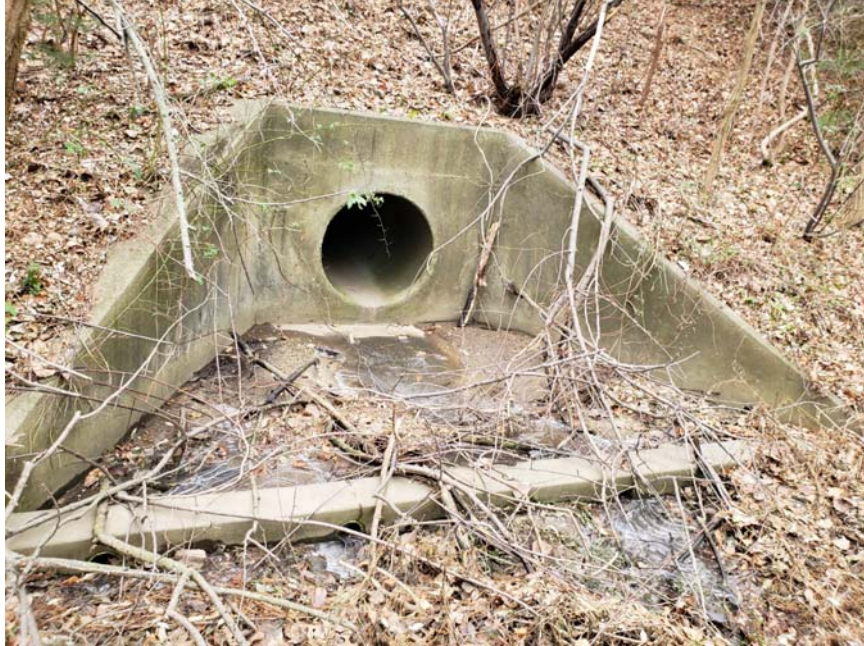
Some siltation and debris- RB#284
