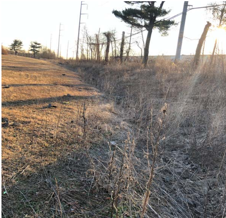
Siltation, vegetative growth and debris- DS#5
