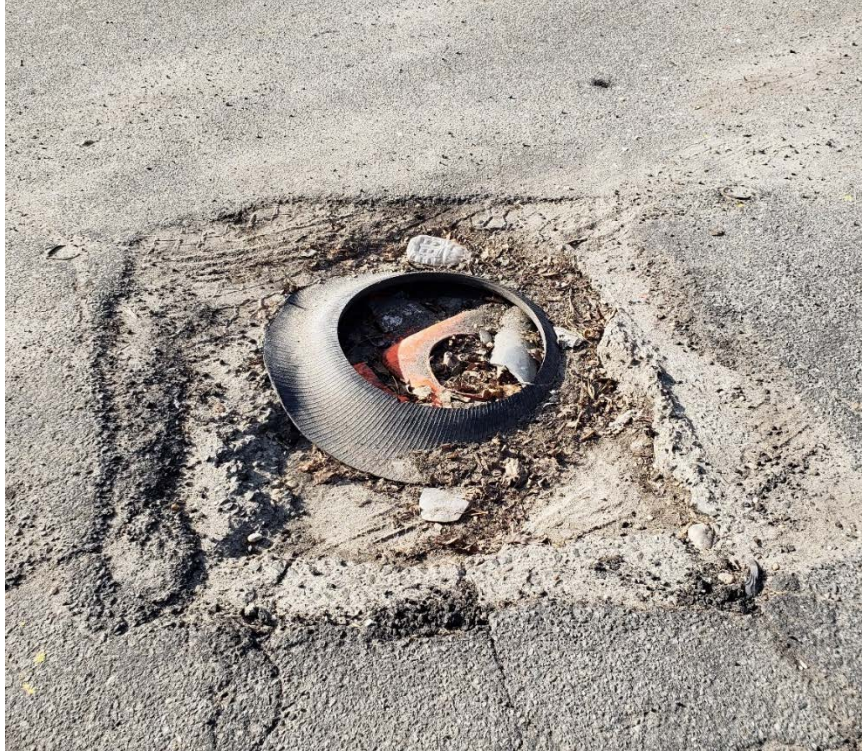
Well Broken at Grade – SE-2
