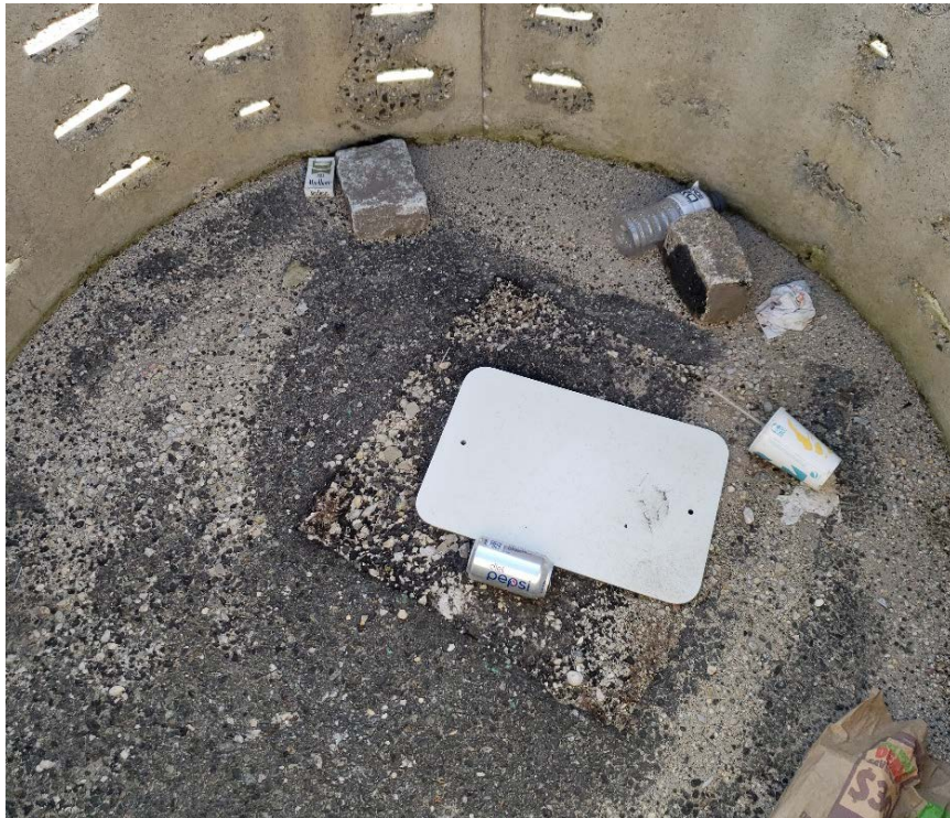
Well Broken at Grade – R-18
