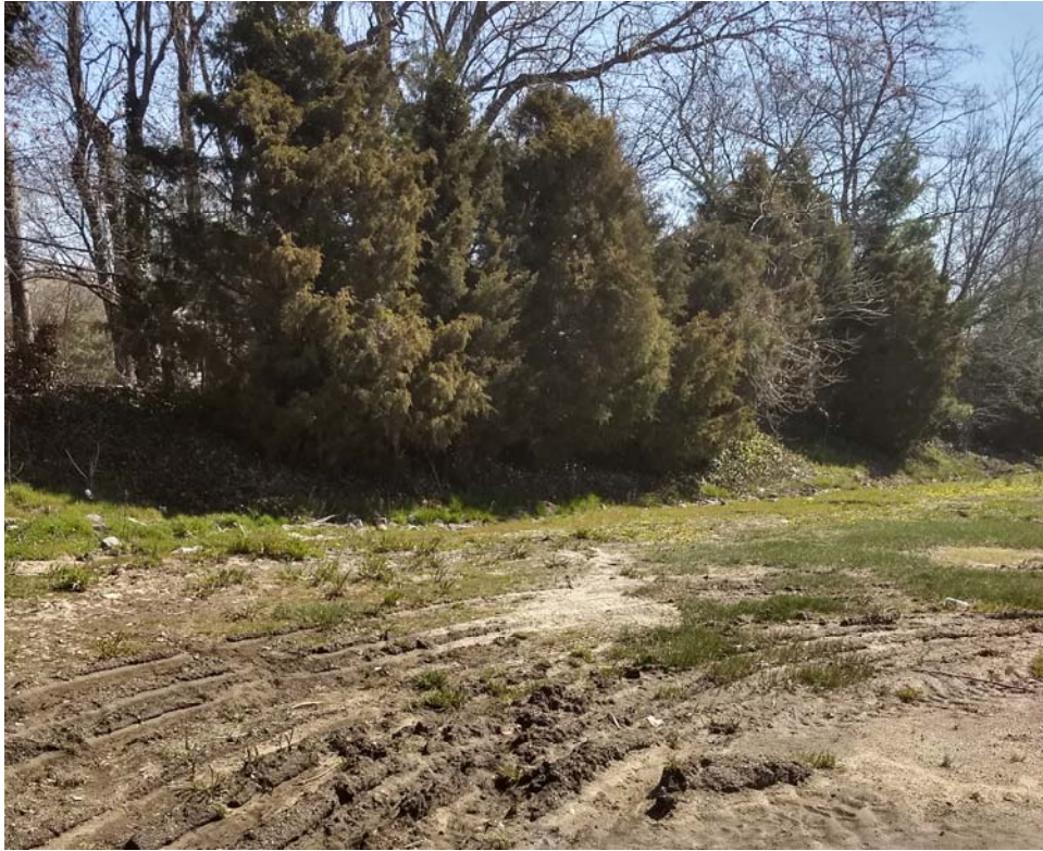
Vegetative surface erosion in Area C
