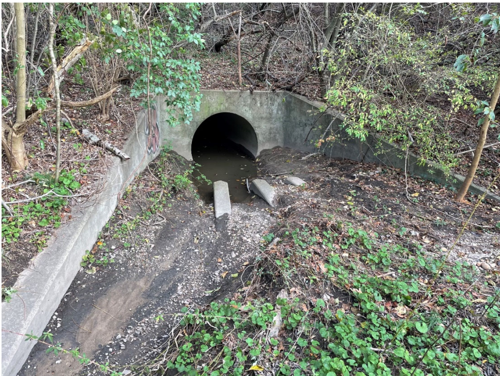
Siltation, Debris, and Vegetative Growth – HW#1 in RB#571
