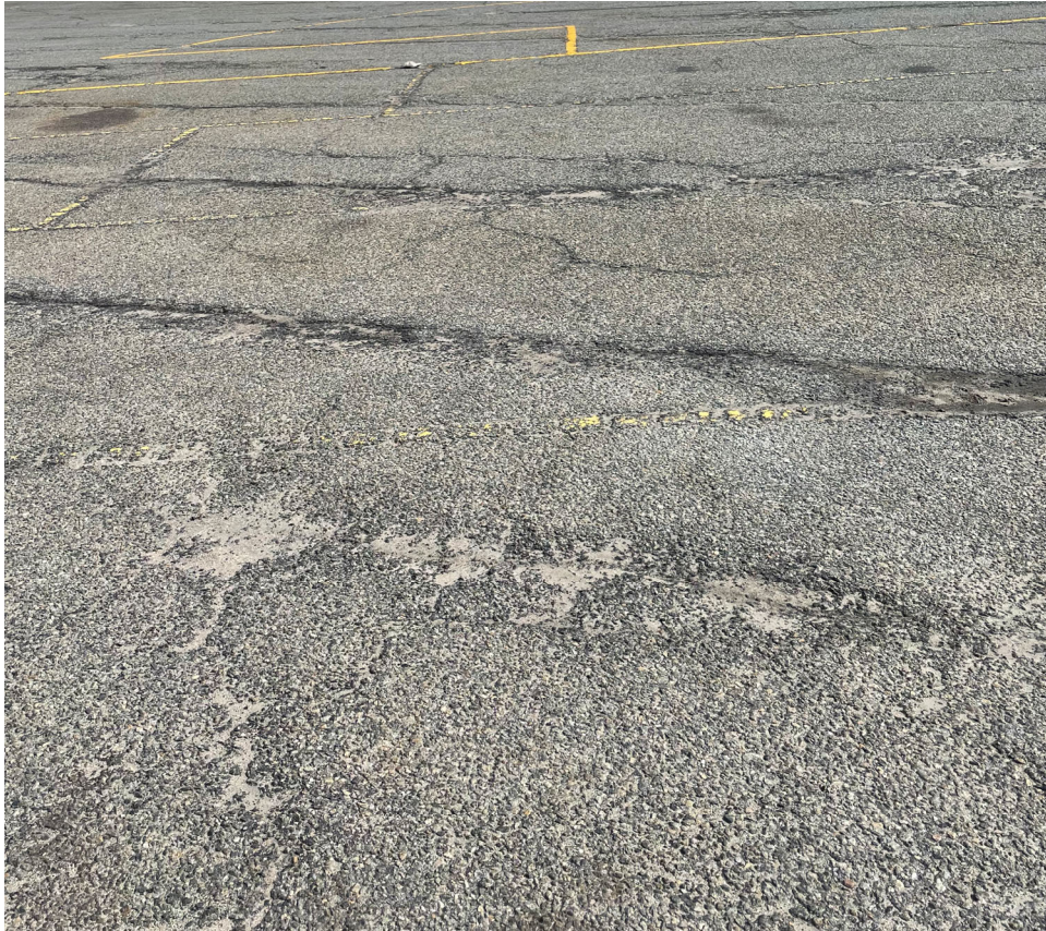
Minor Surface Cracks in Area D
