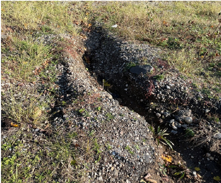
Vegetative Cover Erosion in Area B
