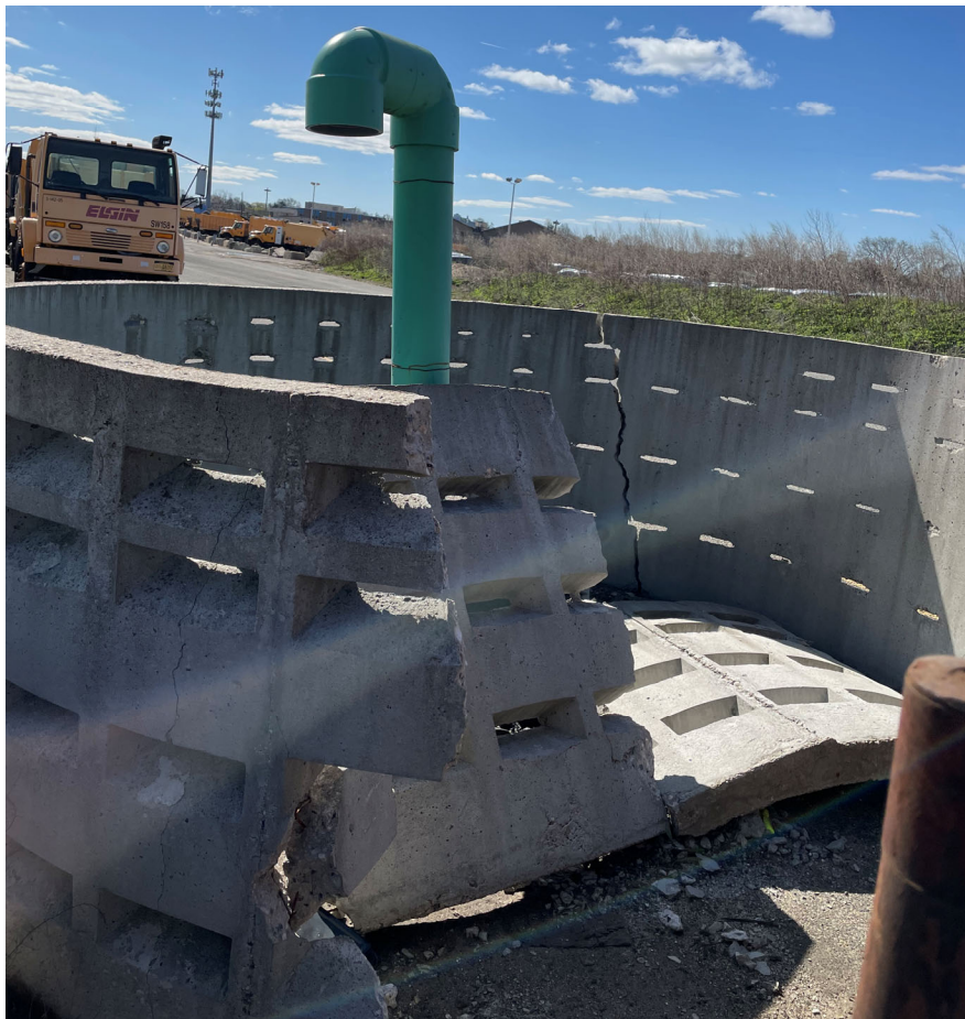
Broken Protective Concrete Ring – R-13
