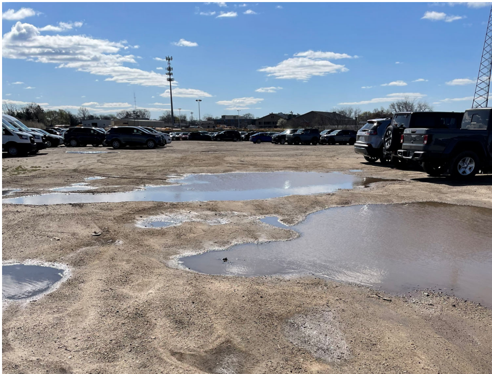
Ponding in Area A
