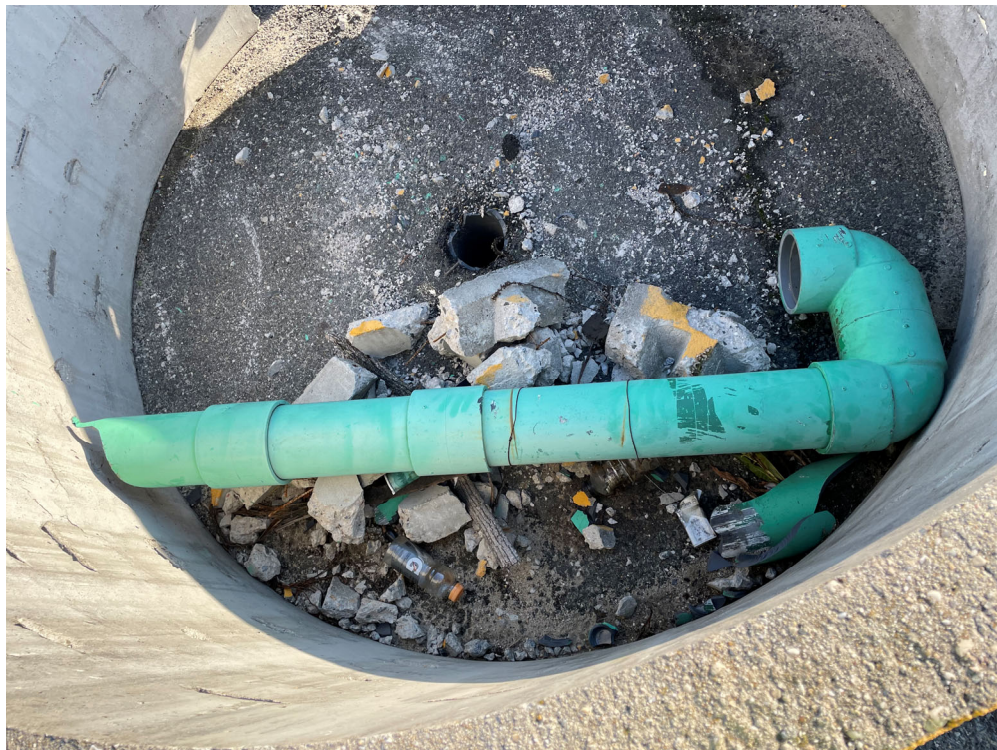
Well Casing Broken at Grade – R-22
