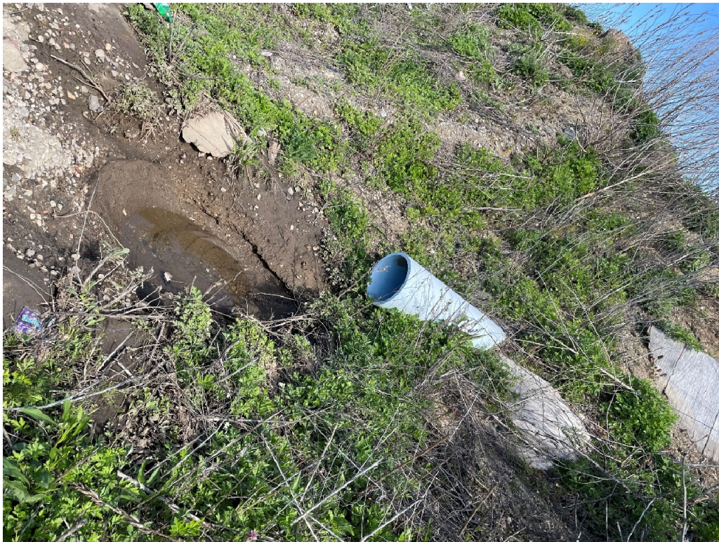
Erosion from drainpipe in DS #6
