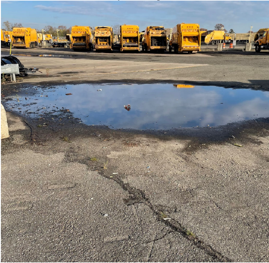
Ponding in Area E
