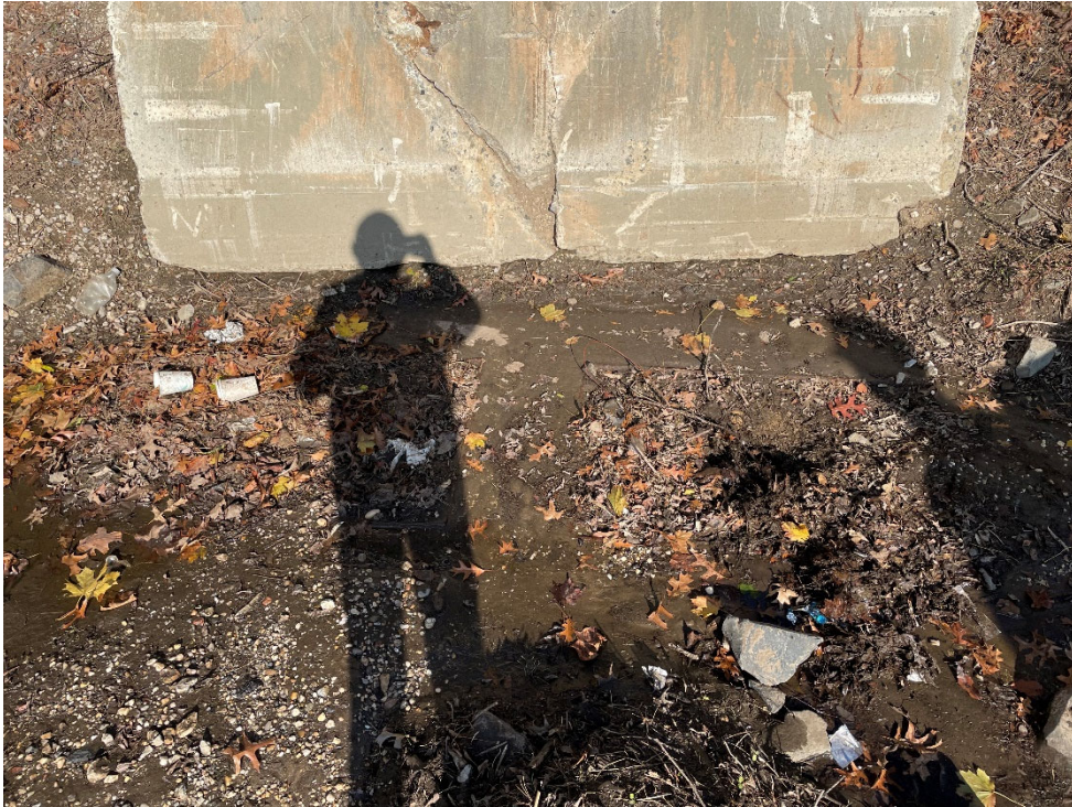
Catch Basin #5 Covered with Sediment and Debris
