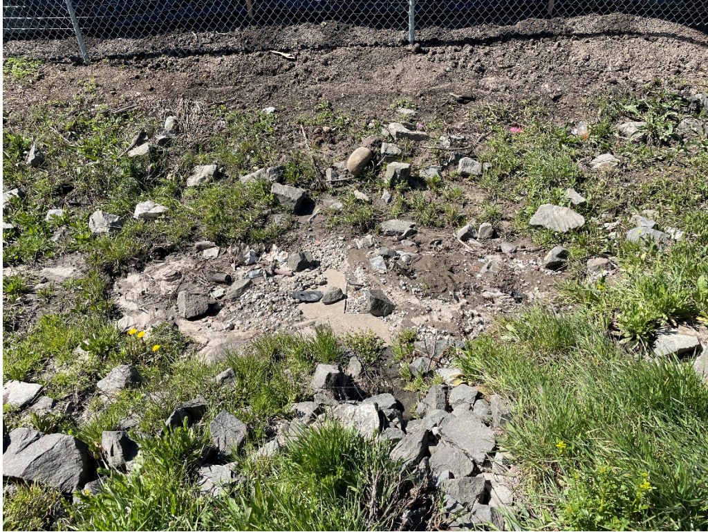
Grate Covered with Sediment and Debris – CB #2
