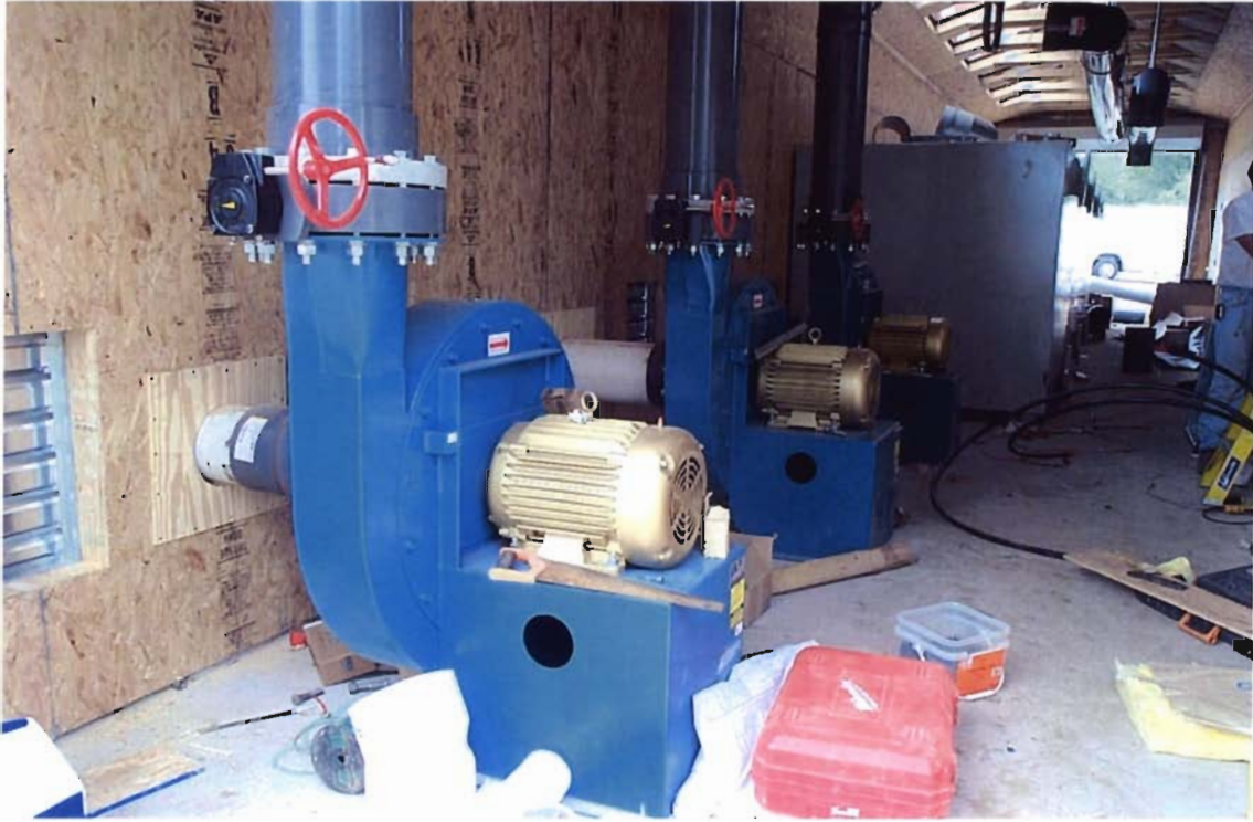
Photograph 8: Centrifugal blowers in equipment building.
