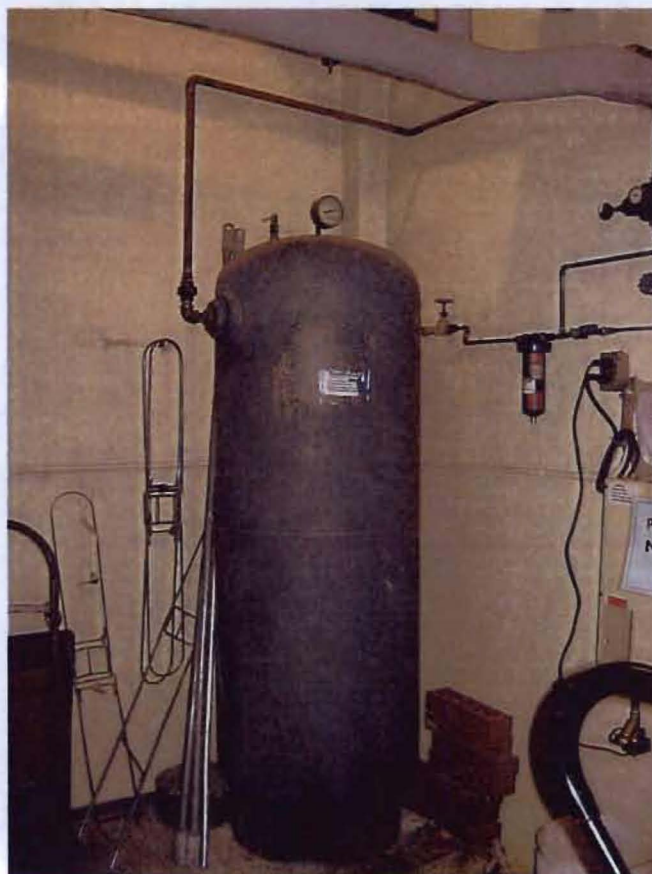
WC – Oil Tank (SB1)
