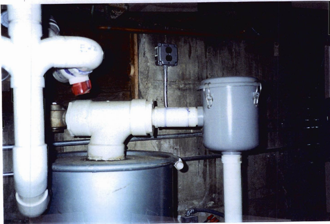
5. Piping from SVES moisture separator feeding the particulate filter
