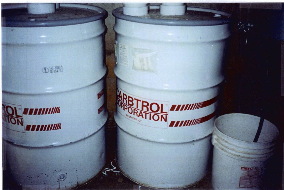
6. SVES air purification canisters in the basement of Atlas Graphics site
