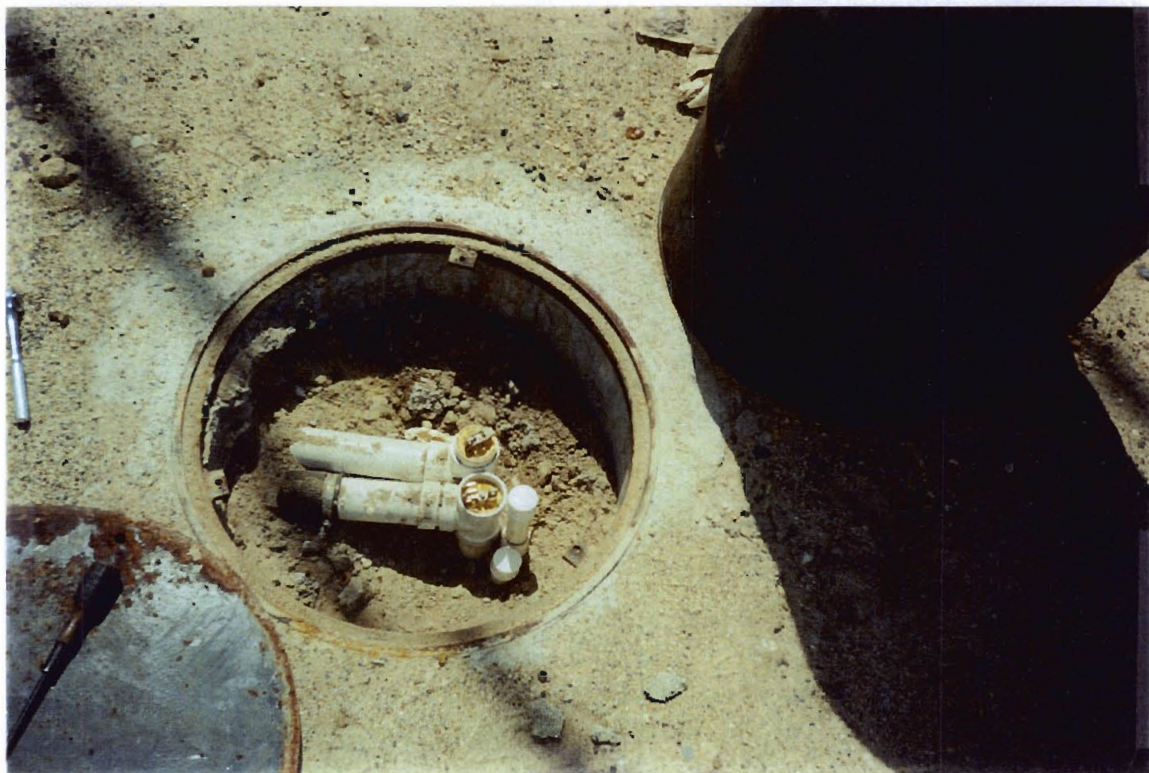
1. Manway providing access to tops of extraction wells and sparge points
