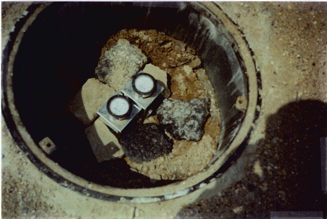
9. SVES extraction well flow meters inside manway at west parking area of site
