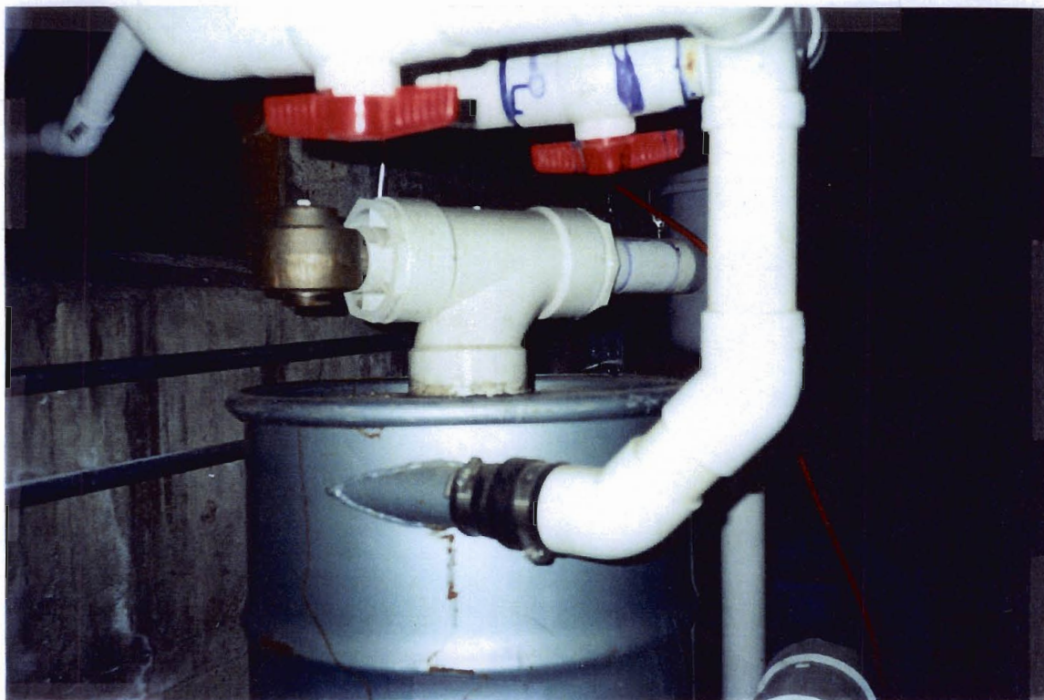
13. Input to SVES moisture separator from manifold and output to particulate filter
