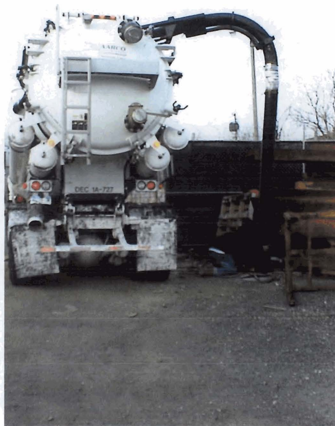
2. Active cleanout of the secondary cesspool "SCP-02", January 24, 2008.
