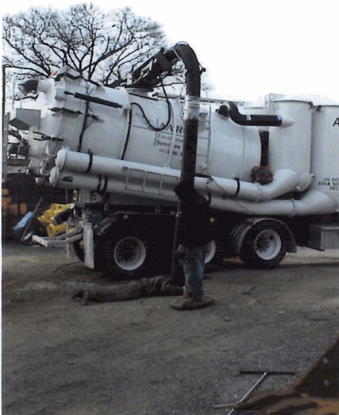
1. Active cleanout of the primary cesspool "PCP-01", January 24, 2008.
