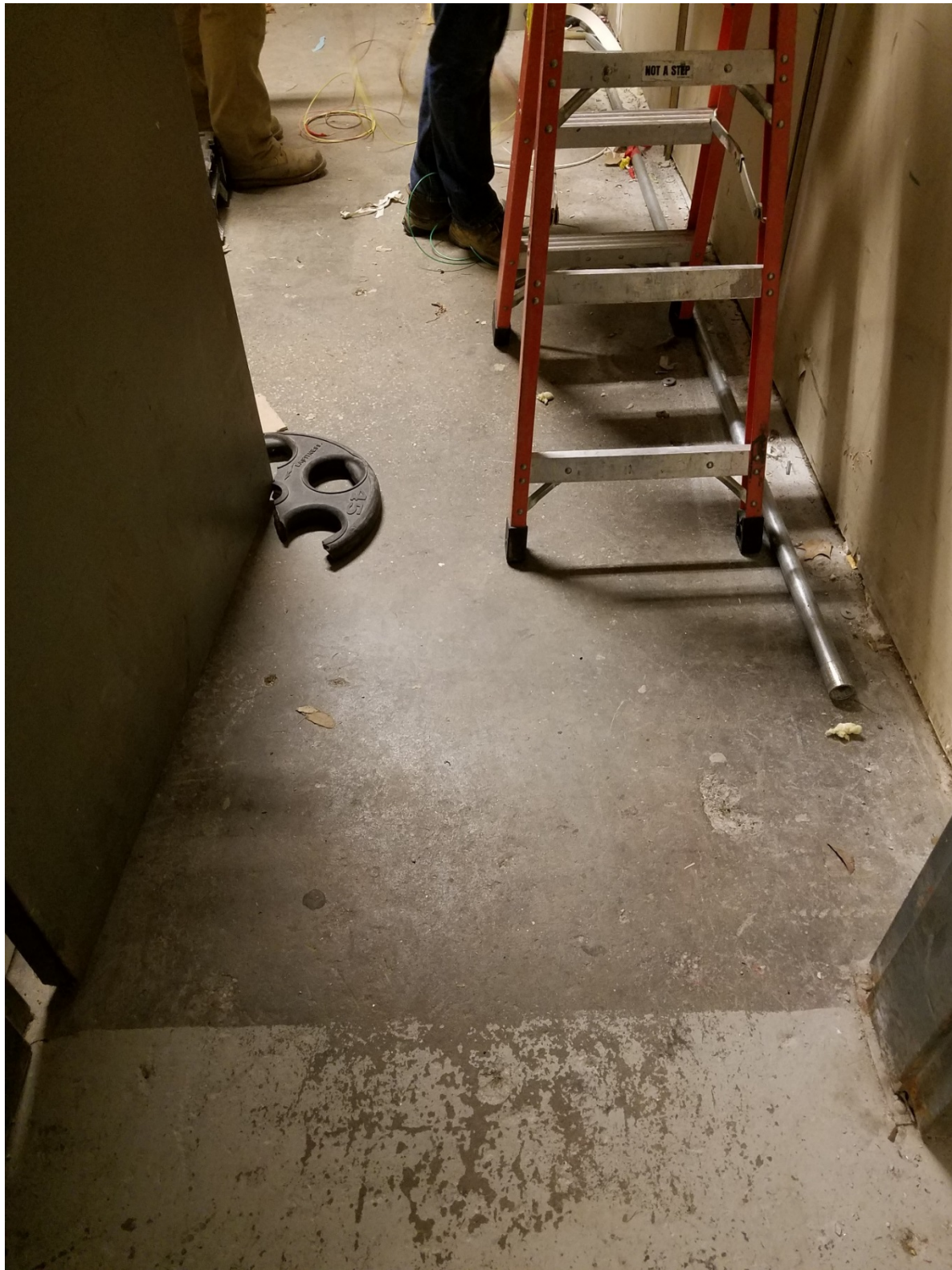
Storage Room Floor Condition – Facing North
