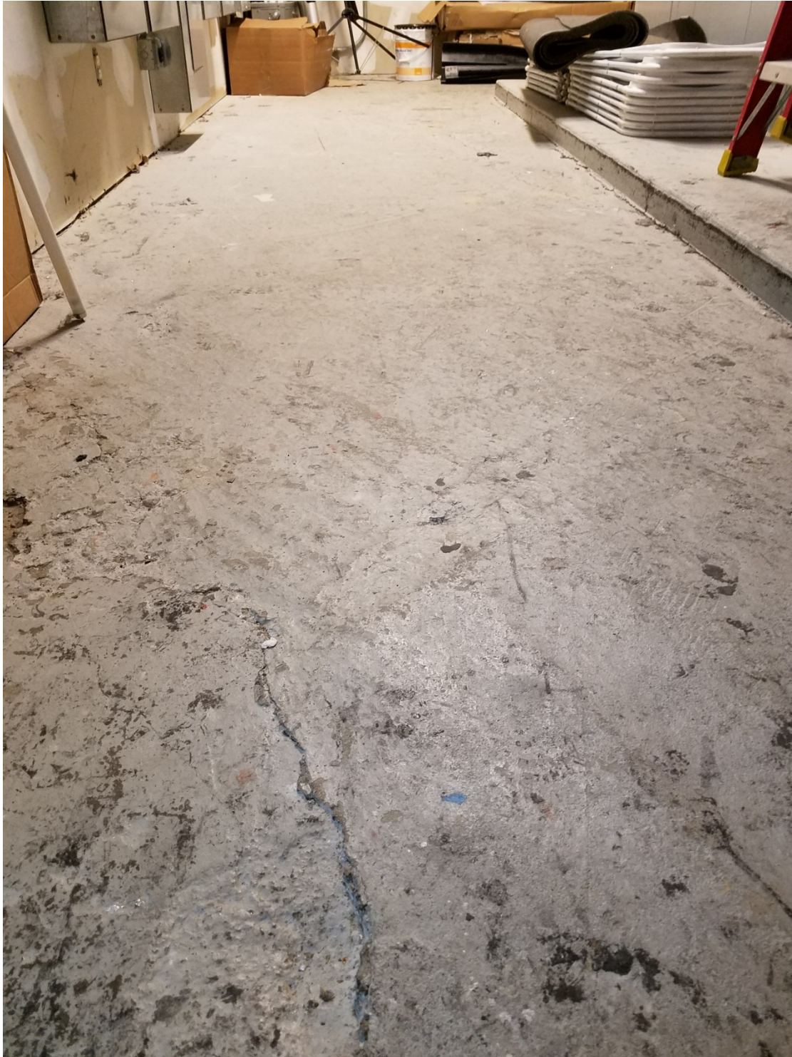
Electrical Room Floor Condition – Facing North
